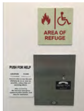
Two-way communication phone for area of refuge
