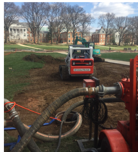
Stormwater management and spill response on McKeldin Mall.
