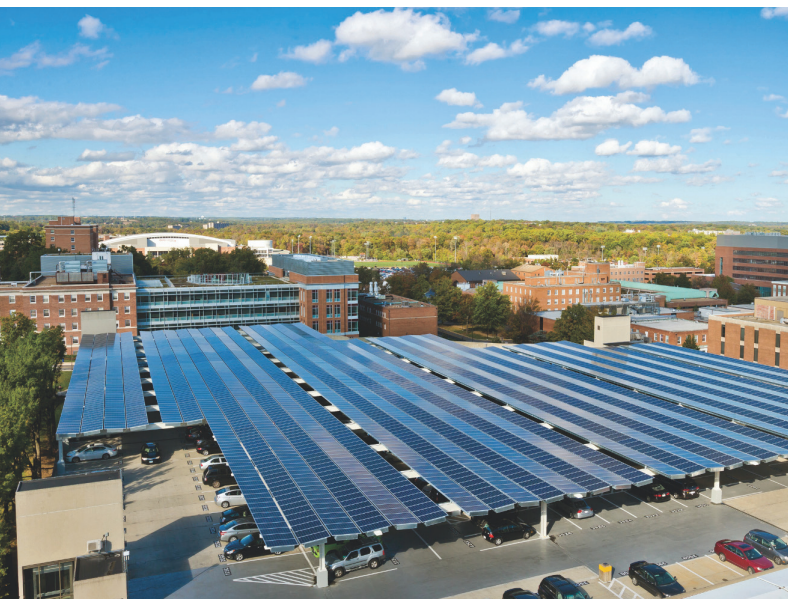
Solar panels on the Regents lane parking garage
