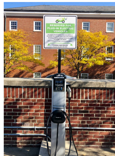
Electric vehicle charging station
