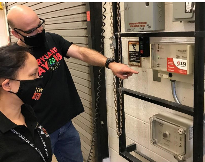
An OFM Fire Protection Engineer (front) witnesses the Flamex acceptance test The Clarice scene shop staff
