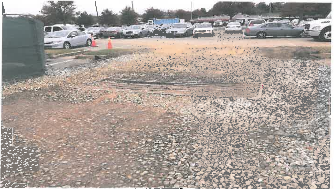
Photo 8. Sediment laden Stabilized Construction Entrance 2 Exit to the Car Park
