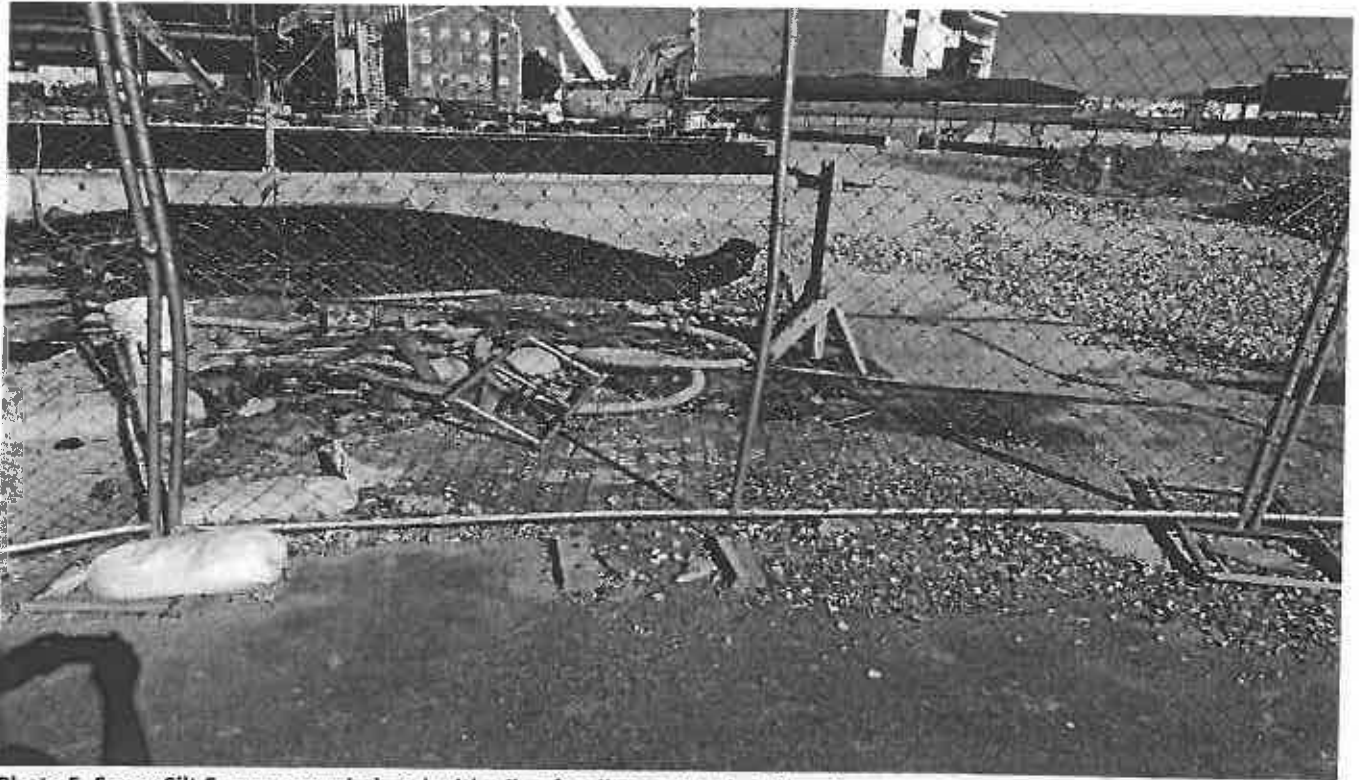
Photo 5. Super Silt Fence overwhelmed with pile of sediment North of the site
