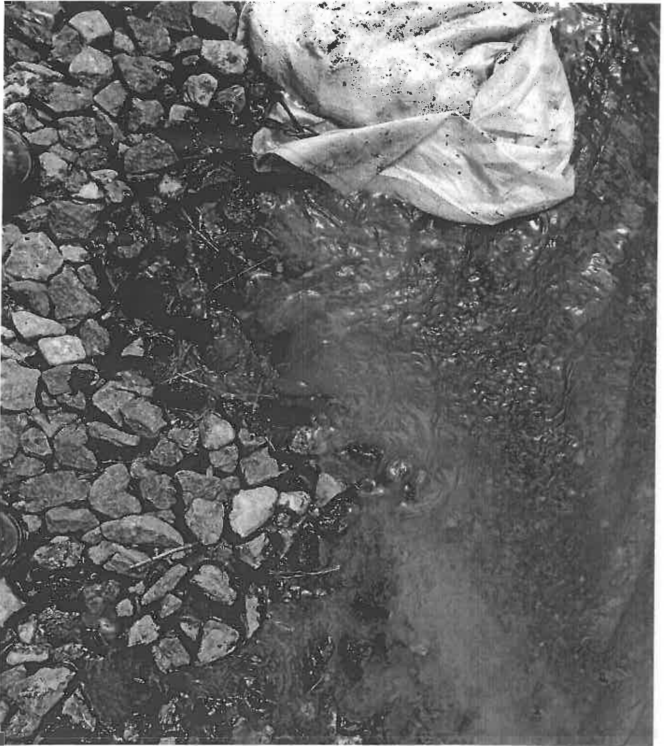
Photo 11. Sediment laden runoff from site to stormdrain on Cole Field Drive in photo 1 off the site.
