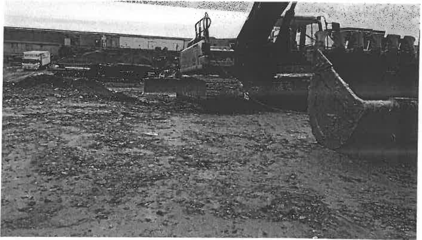
Photo 14. Stabilized Construction Entrance with little or no stones despite ongoing rain event.
