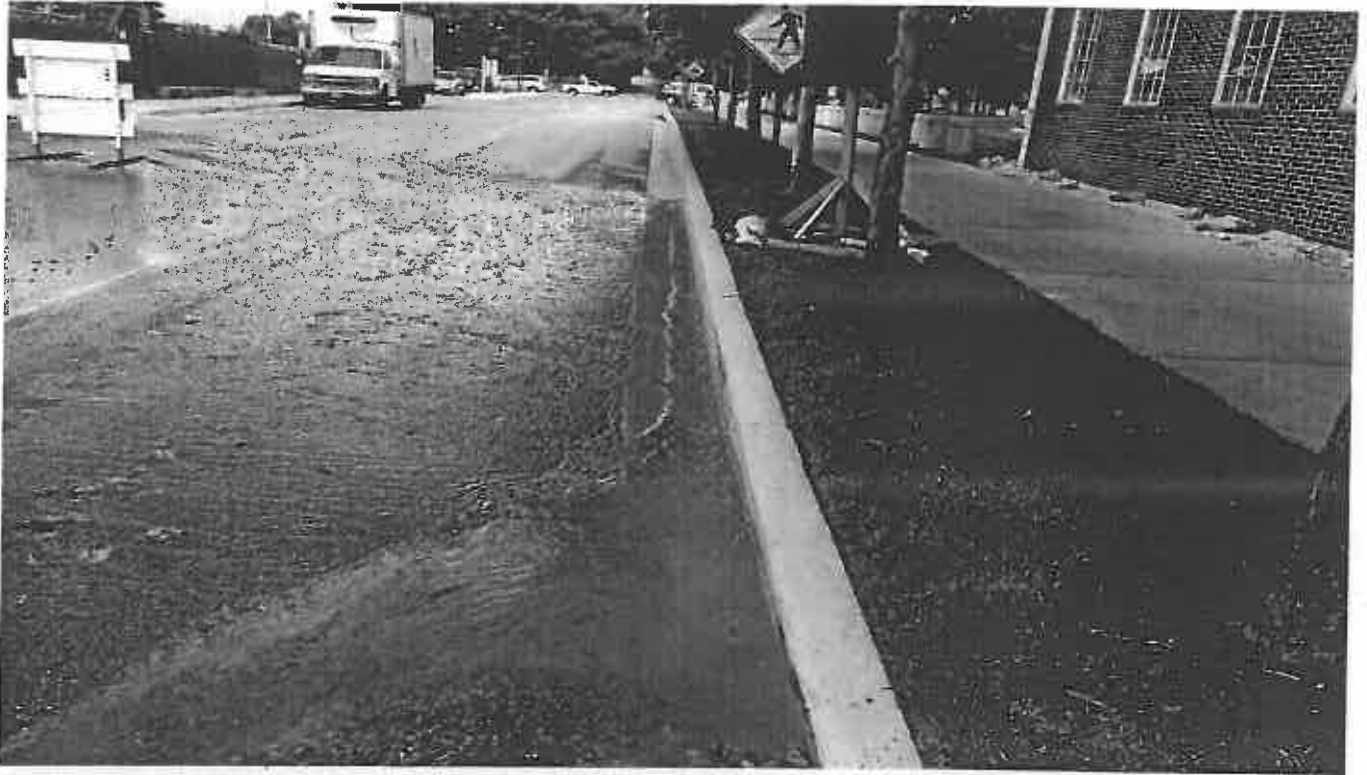
Photo 1. Ongoing pumping of Sediment laden stormwater into stormdrain on Cole Fieldhouse Drive NW off site
