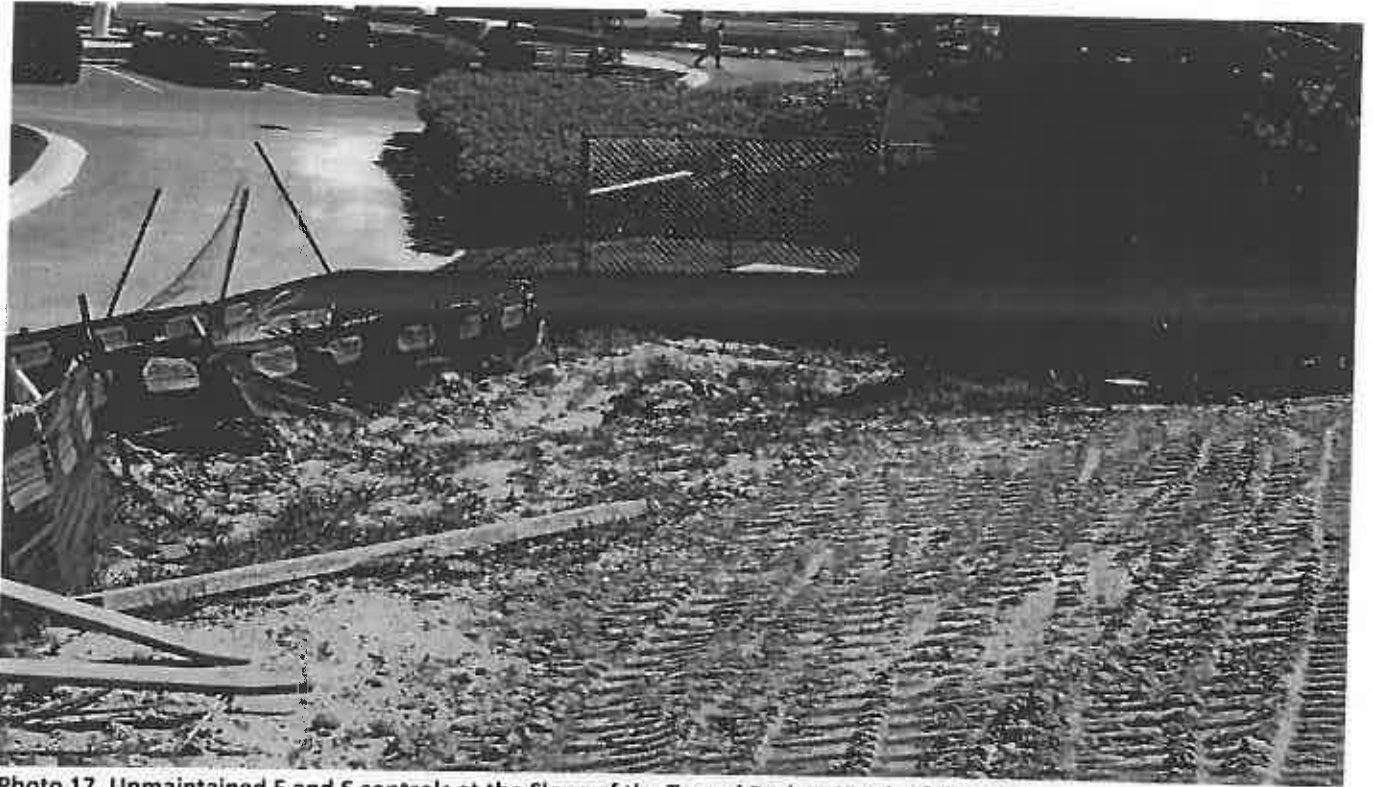
Photo 17. Unmaintained E and S controls at the Slope of the Tunnel Project North of the Site
