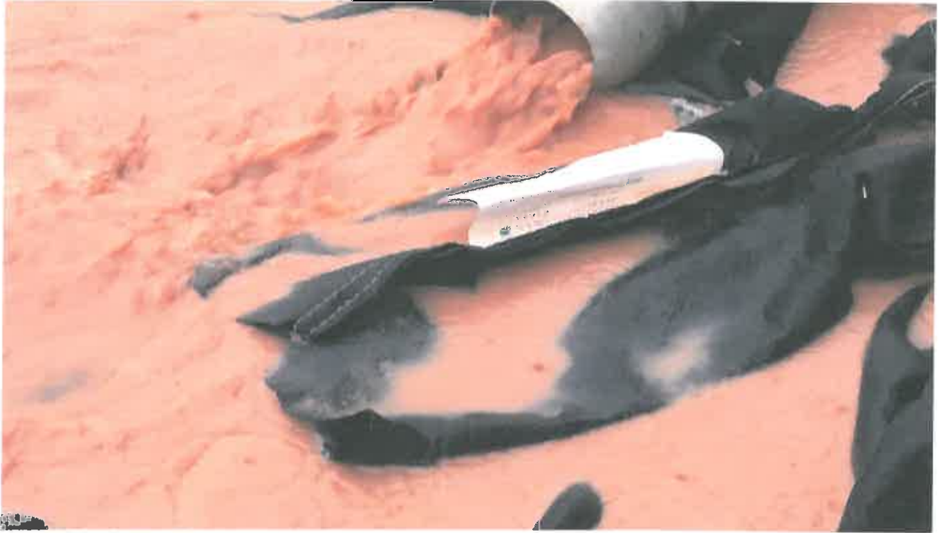
Photo 3. Ongoing pumping of Sediment laden Stormwater into active stormdrain onsite (State Waters)
