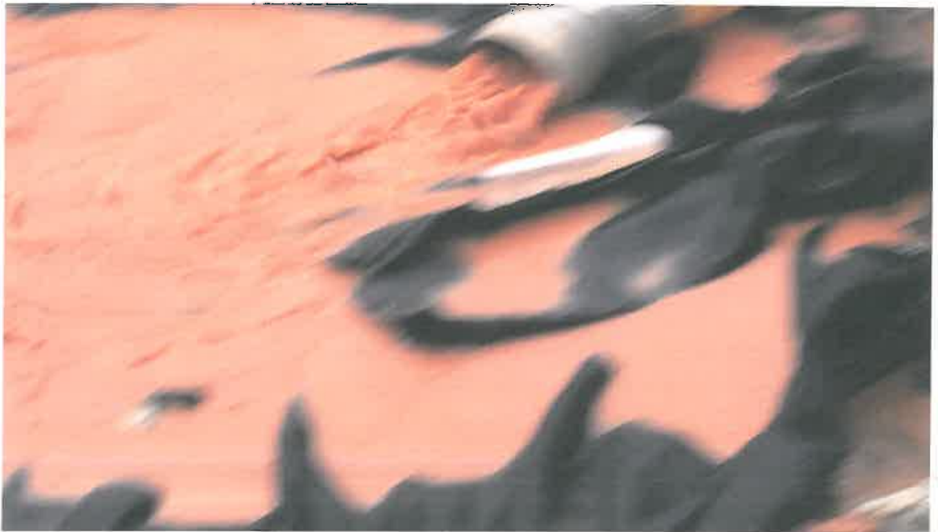
Photo 2. Ongoing pumping of Sediment laden Stormwater into active stormdrain onsite (State Waters)
