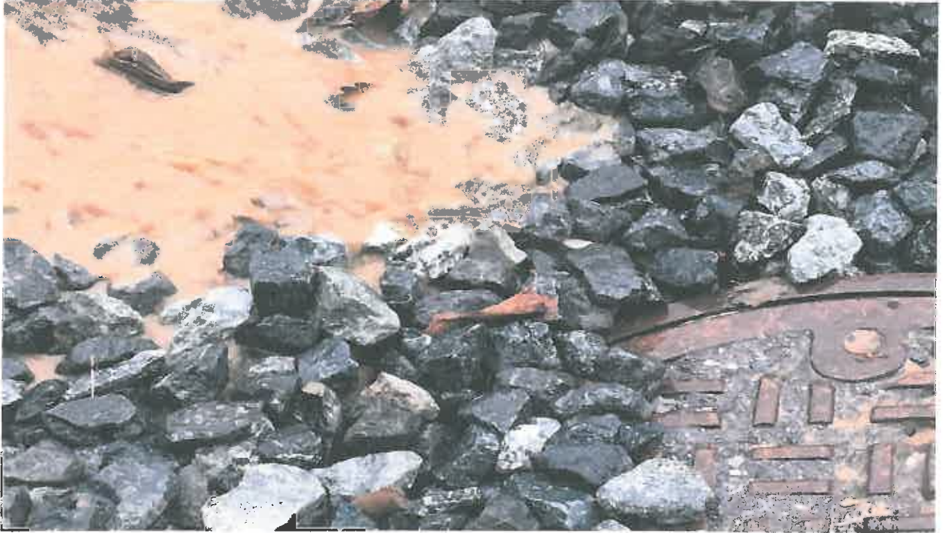
Photo 11. Ongoing pumping of Sediment laden Stormwater into active stormdrain onsite (State Waters)
