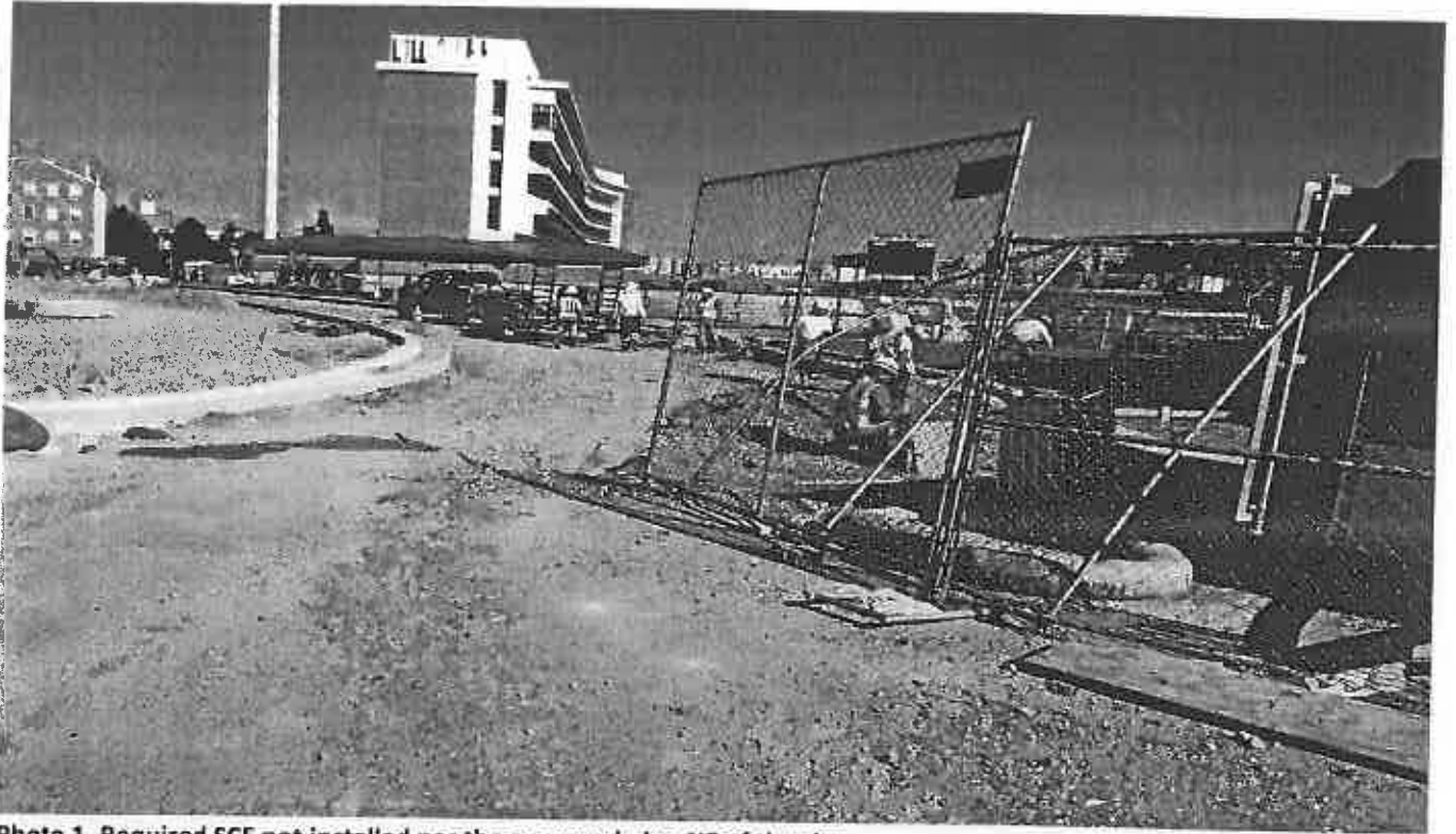
Photo 1. Required SCE not installed per the approved plan NE of the site.
