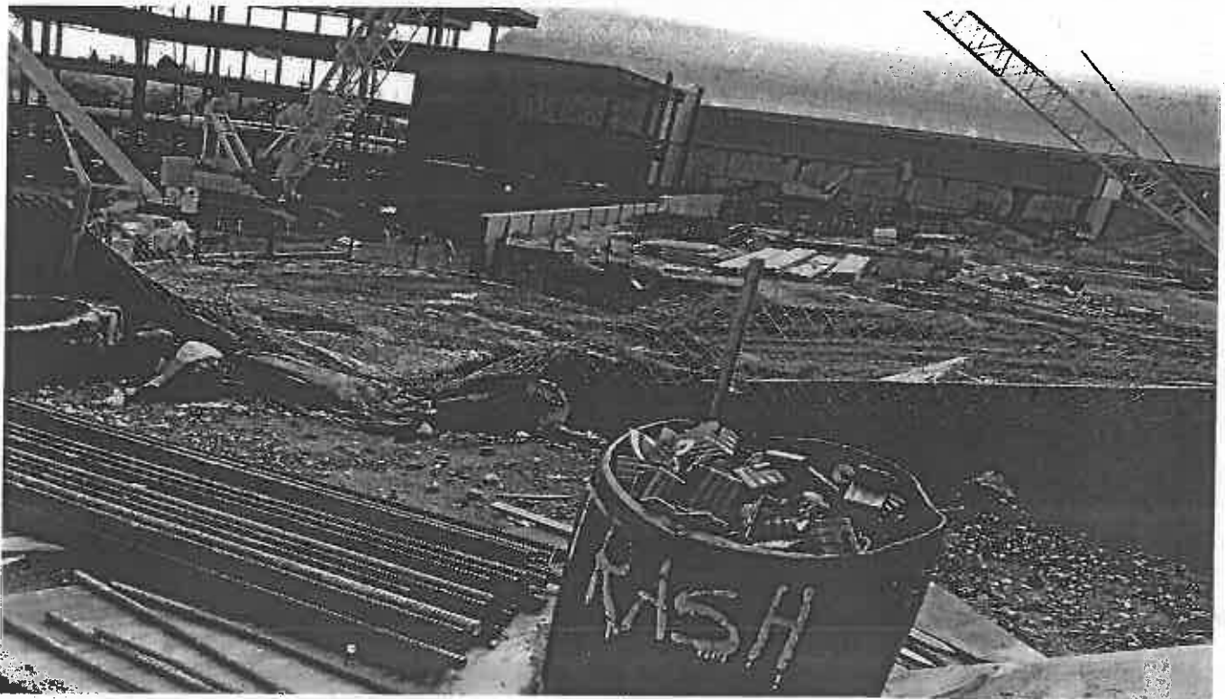
Photo 2. View of the deficient erosion and sediment control South of the site
