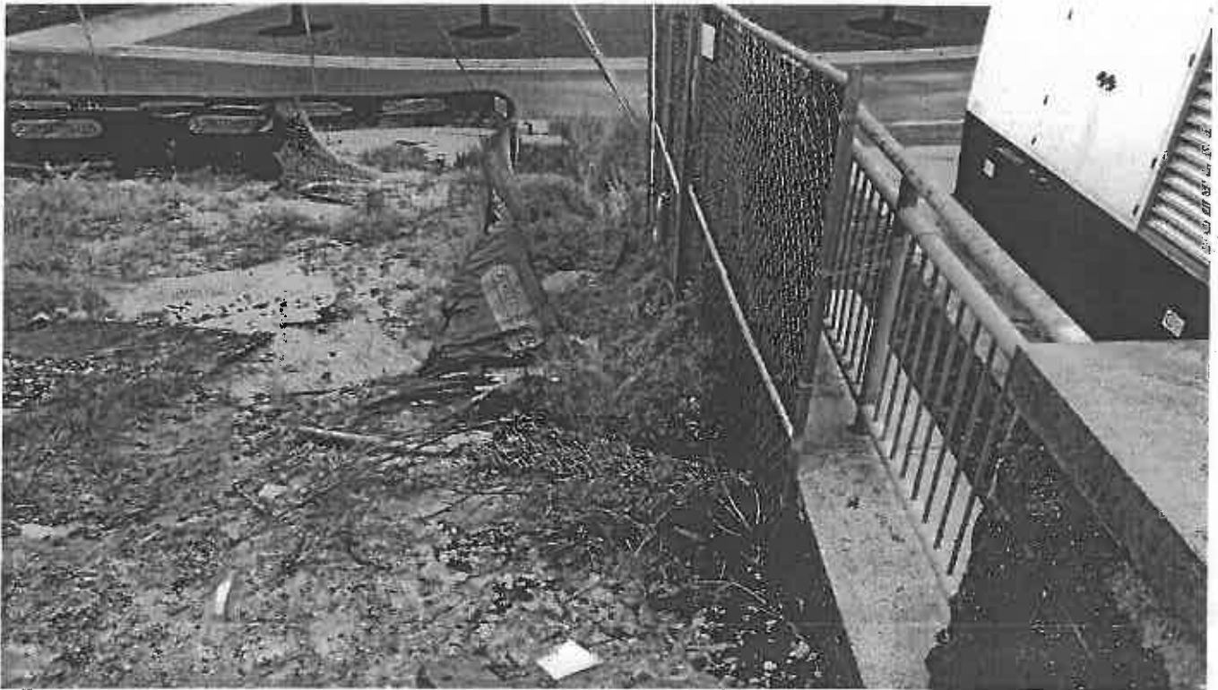
Photo 8. Unmaintained E and S controls at the Slope of the Tunnel Project North of the Site
