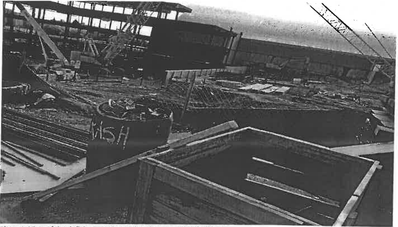
Photo 1. View of the deficient erosion and sediment control South of the site
