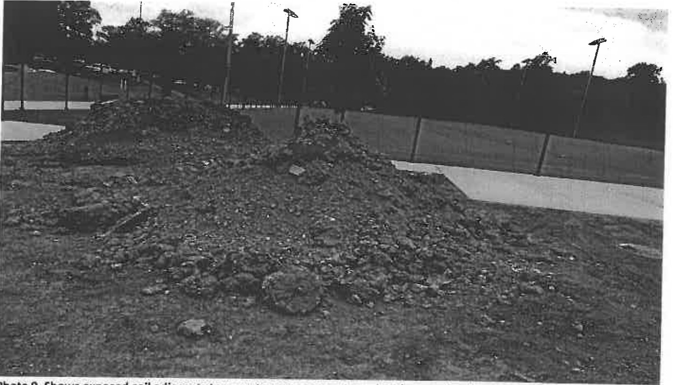
Photo 9. Shows exposed soil adjacent storm water management pond at the new tennis court
