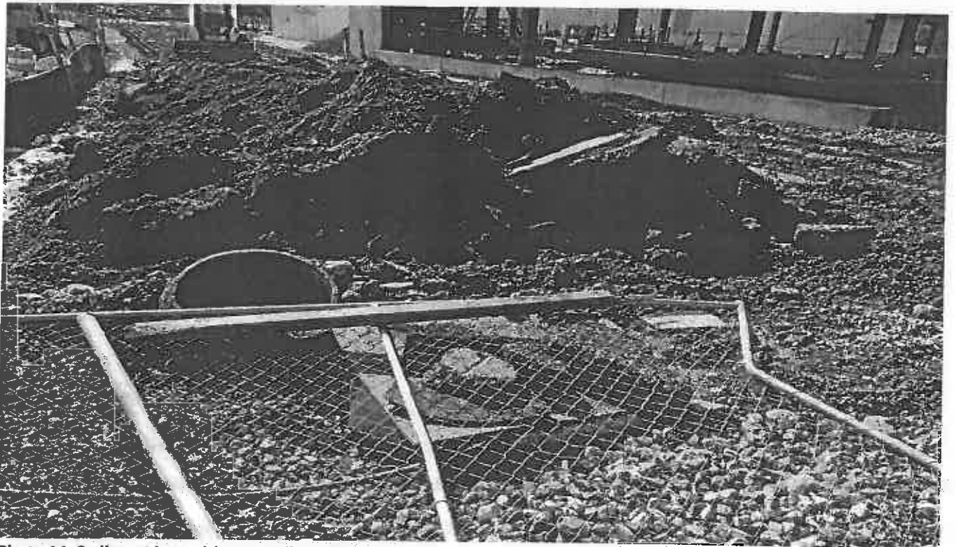
Photo 14. Sediment in position to pollute stormdrain.
