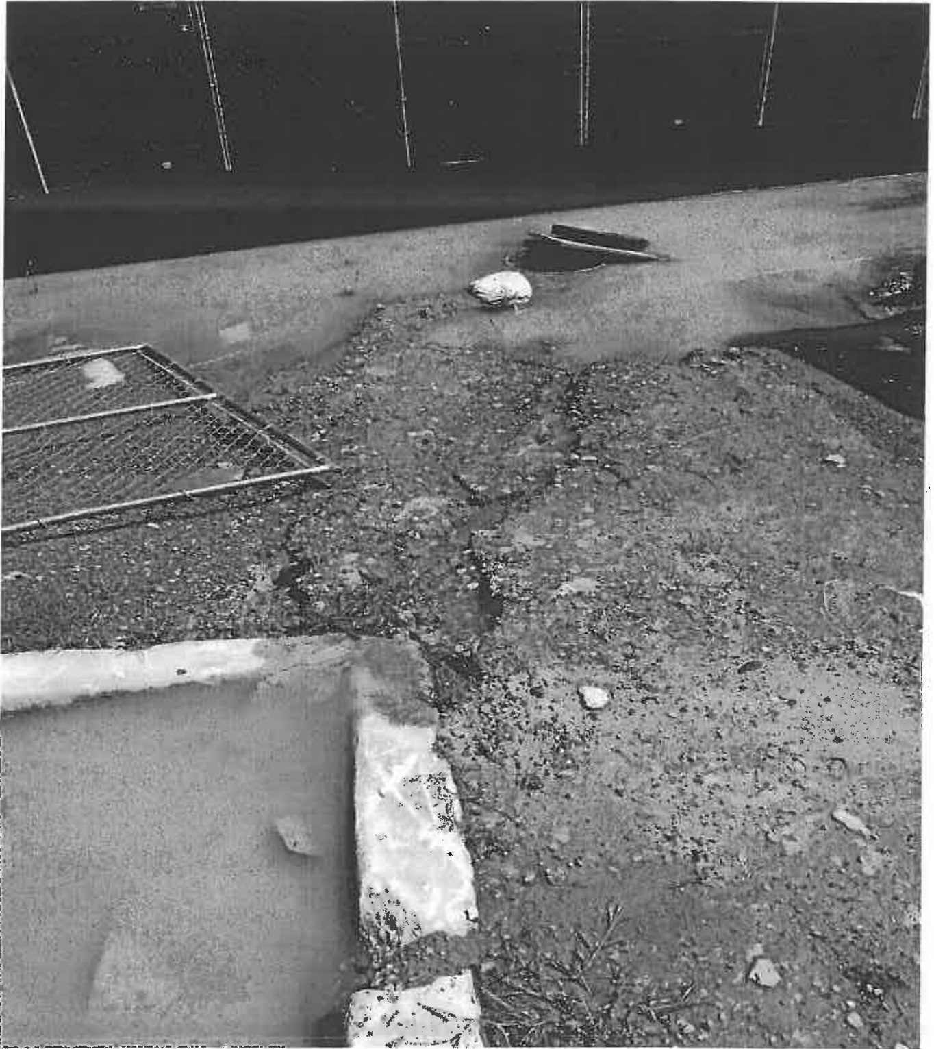
Photo 6. Sediment laden runoff from site to stormdrain on Cole Field Drive in photo 1 off the site.
