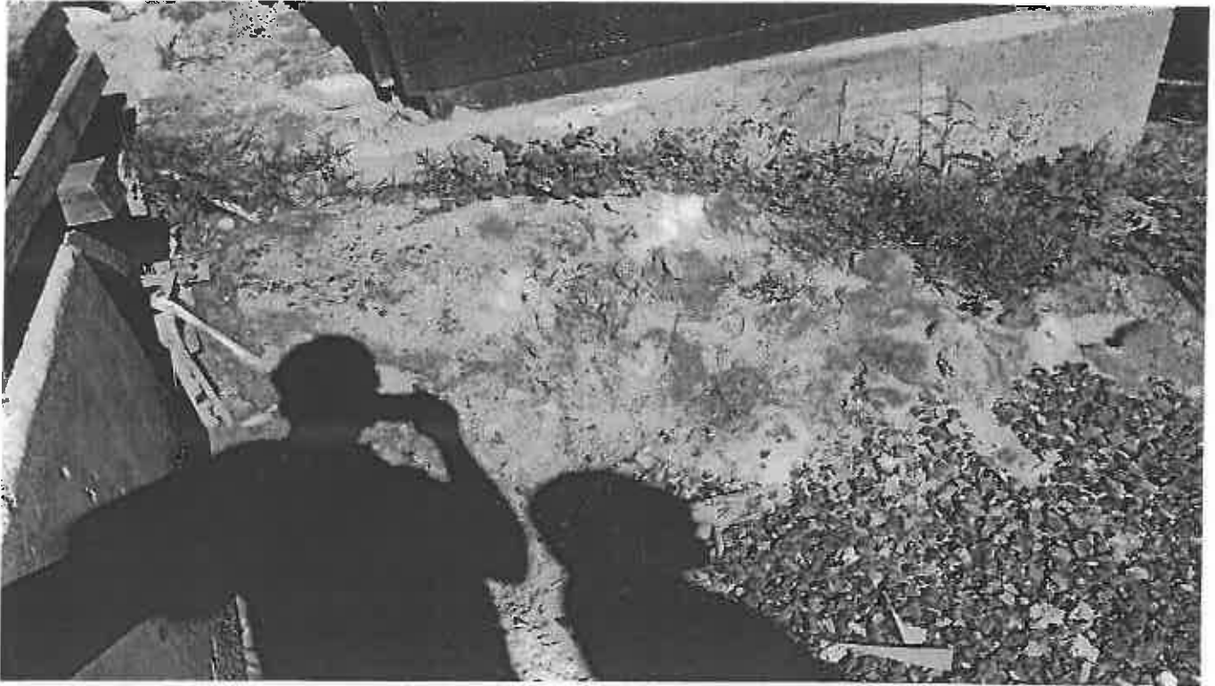
Photo 7. Exposed soil and unmaintained E and S controls at the Slope of the Tunnel Project North of the Site
