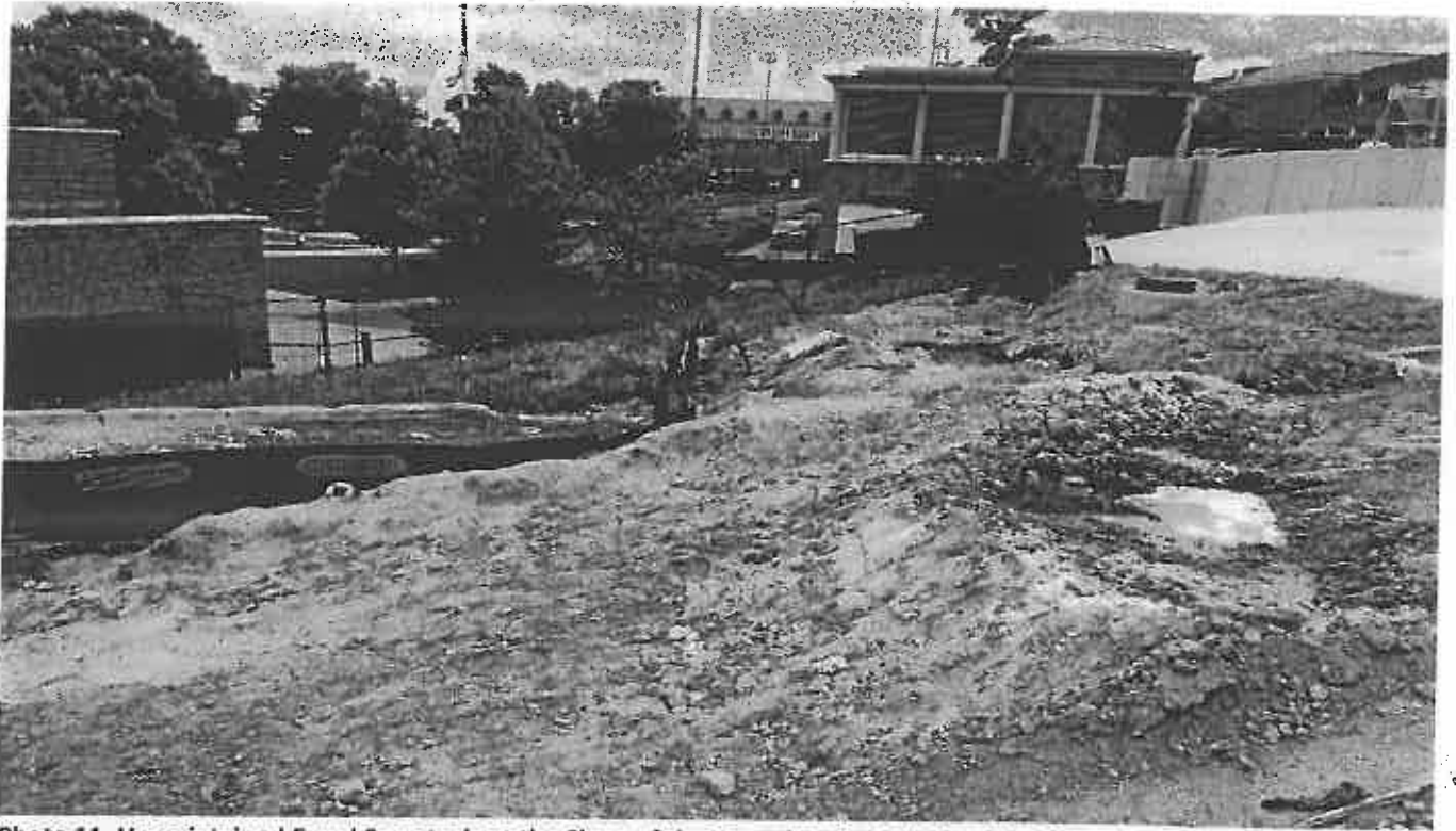
Photo 11. Unmaintained E and S controls at the Slope of the Tunnel Project North of the Site
