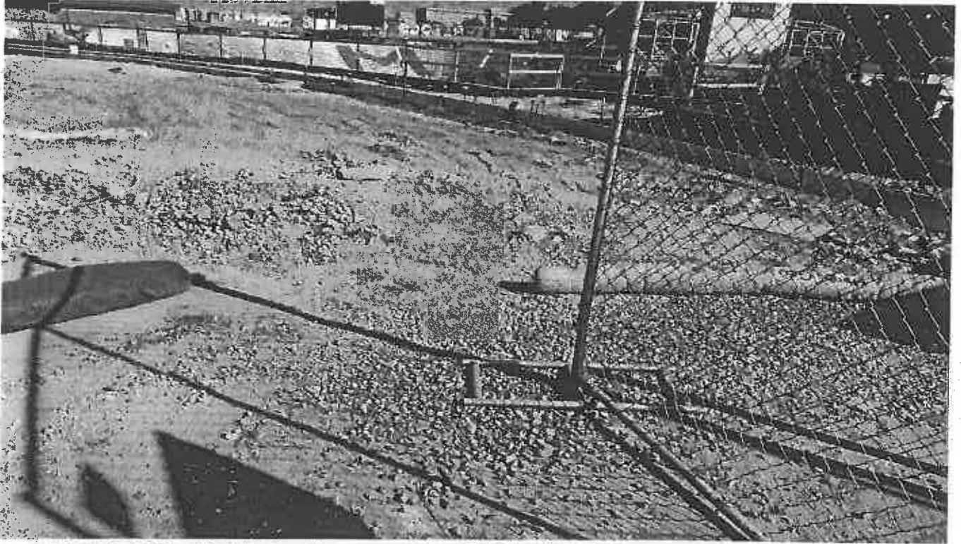
Photo 1. Required SCE not installed per the approved plan NE of the site.
