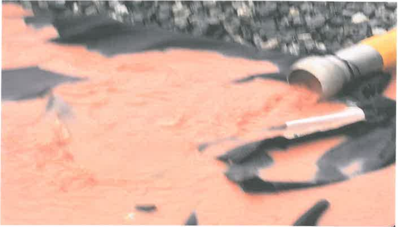
Photo 1. Ongoing pumping of Sediment laden Stormwater into active stormdrain onsite (State Waters)
