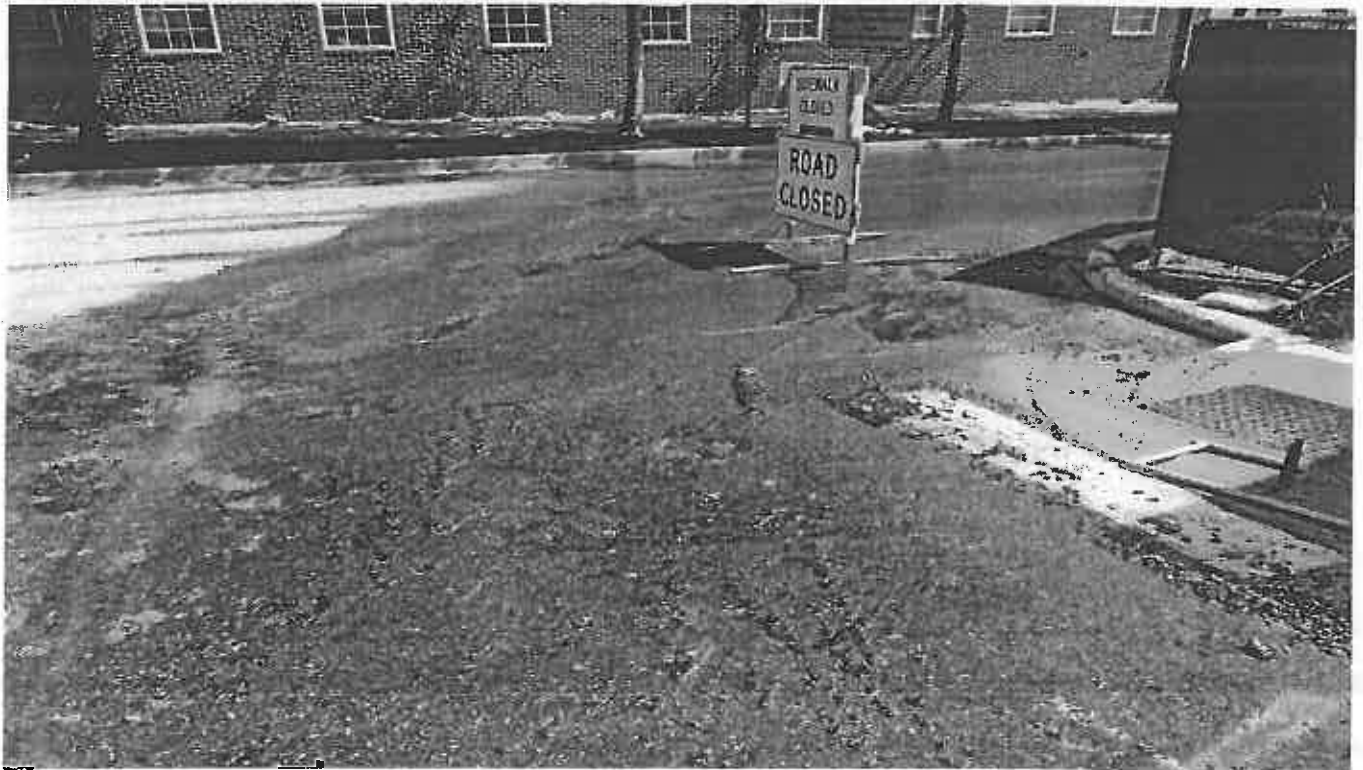
Photo 8. Sediment laden runoff from site to stormdrain on Cole Field Drive in photo 1 off the site.
