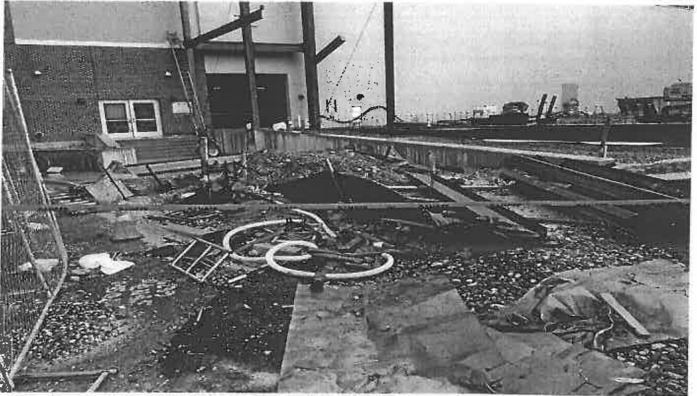
Photo 7. Super Silt Fence overwhelmed with pile of sediment NE of the site
