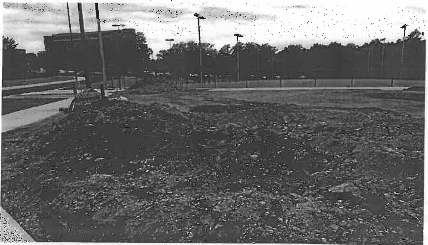
Photo 4. Shows exposed soil adjacent storm water management pond at the new tennis court
