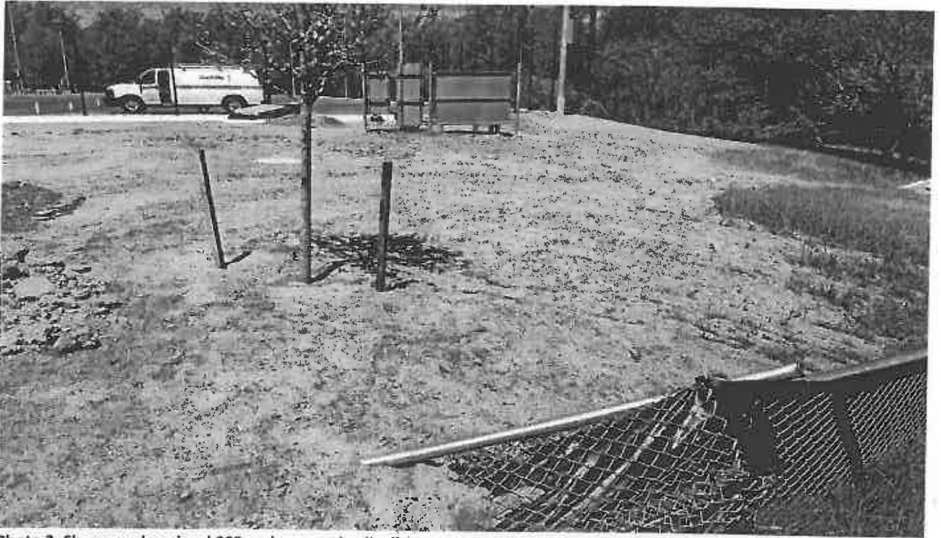
Photo 3. Shows undermined SSF and exposed soil adjacent stormwater management pond at the tennis court
