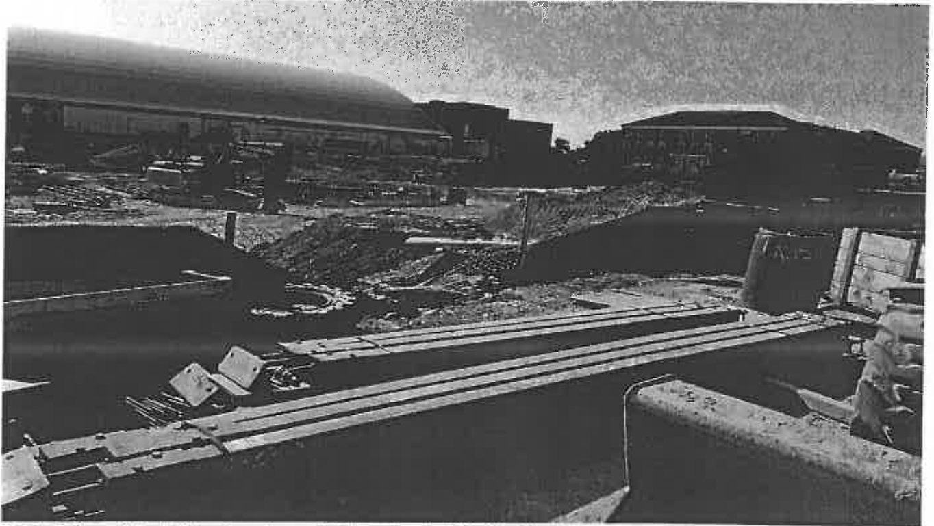
Photo 7. View of the deficient erosion and sediment control South of the site
