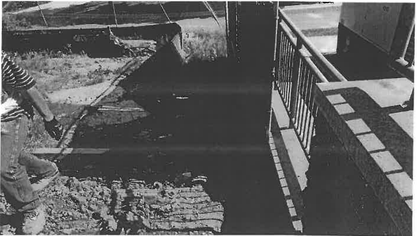
Photo 3. Unmaintained E and S controls at the Slope of the Tunnel Project North of the Site
