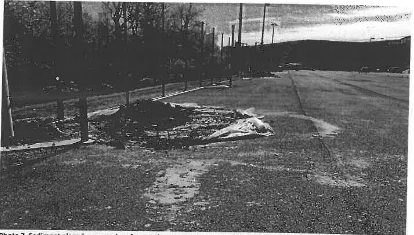
Photo 7. Sediment placed on paved surface at the new tennis court with potentials to impact the stormdrain
