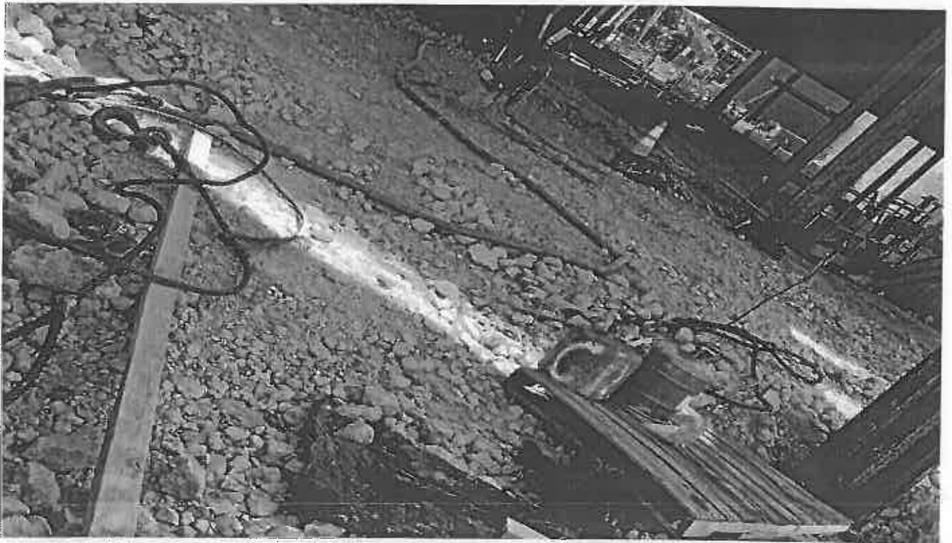
Photo 18. Ongoing pumping of muddy groundwater from foundation footing into active stormdrain onsite.
