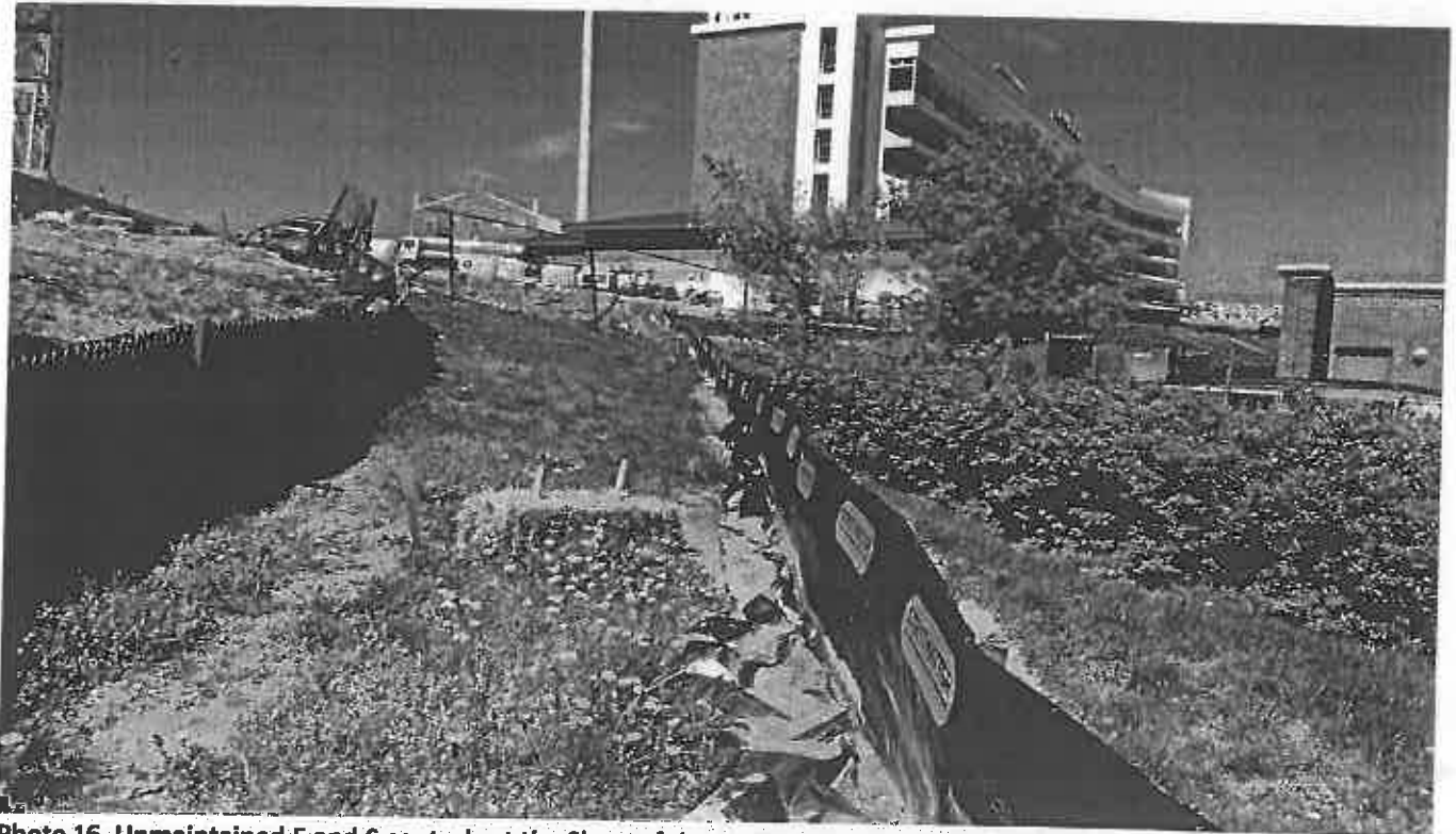
Photo 16. Unmaintained E and S controls at the Slope of the Tunnel Project North of the Site
