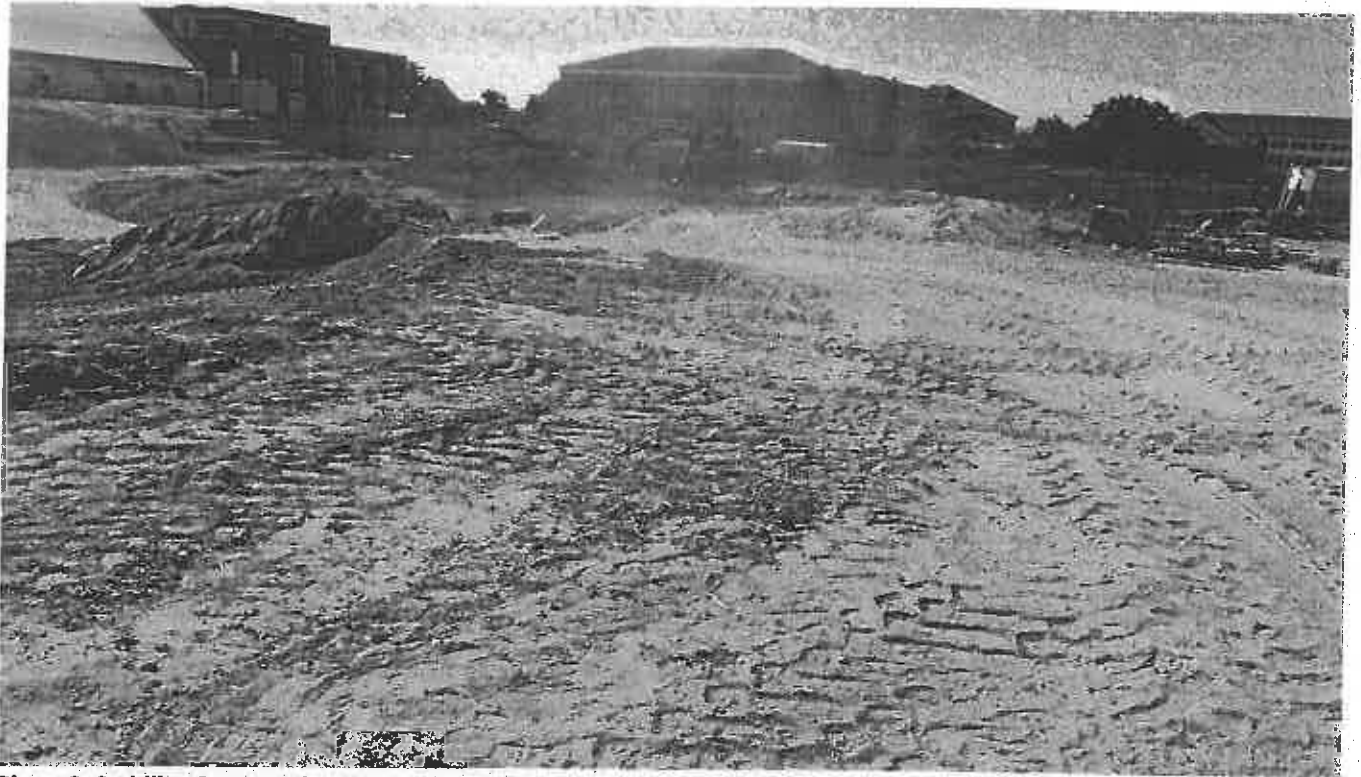
Photo 3. Stabilize Construction Entrance without aggregate stones tracking mud on paved road SW site of site
