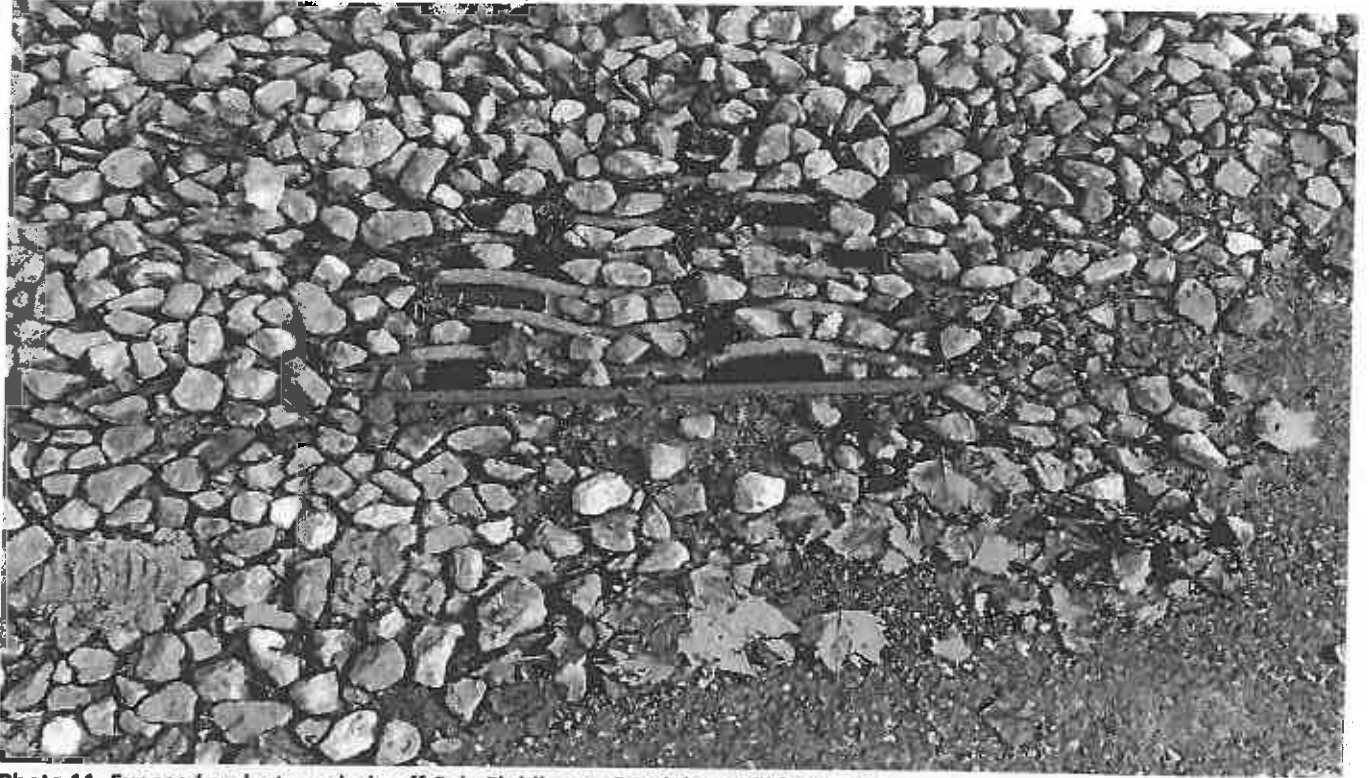
Photo 11. Exposed curb stormdrain off Cole Fieldhouse Road downhill from site
