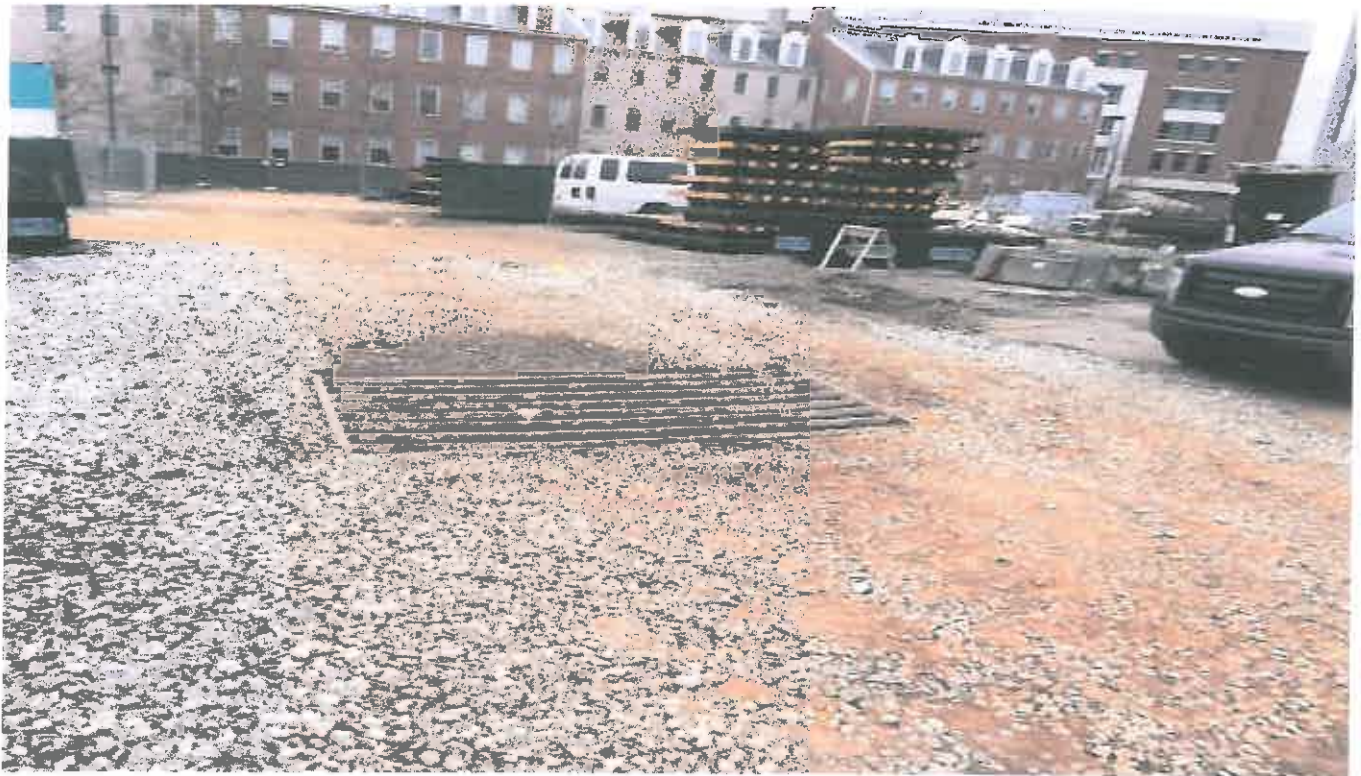
Photo 6. Sediment laden Stabilized Construction Entrance 1 Uphill towards Cole Fieldhouse Drive
