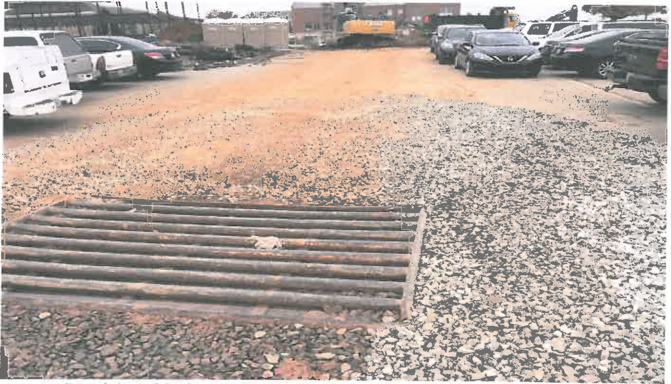
Photo 5. Sediment laden Stabilized Construction Entrance 1 Uphill towards Cole Fieldhouse Drive
