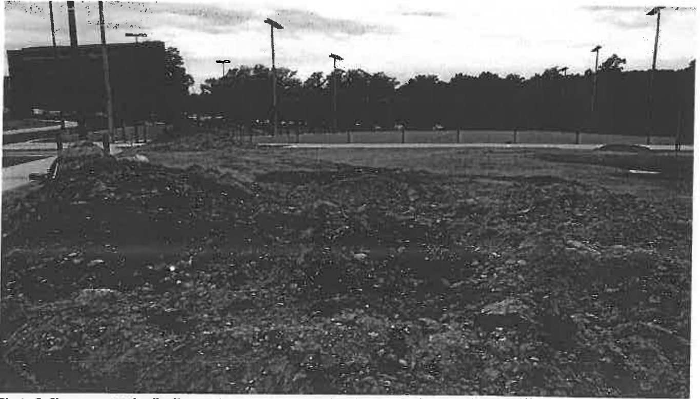
Photo 3. Shows exposed soil adjacent storm water management pond at the new tennis court
