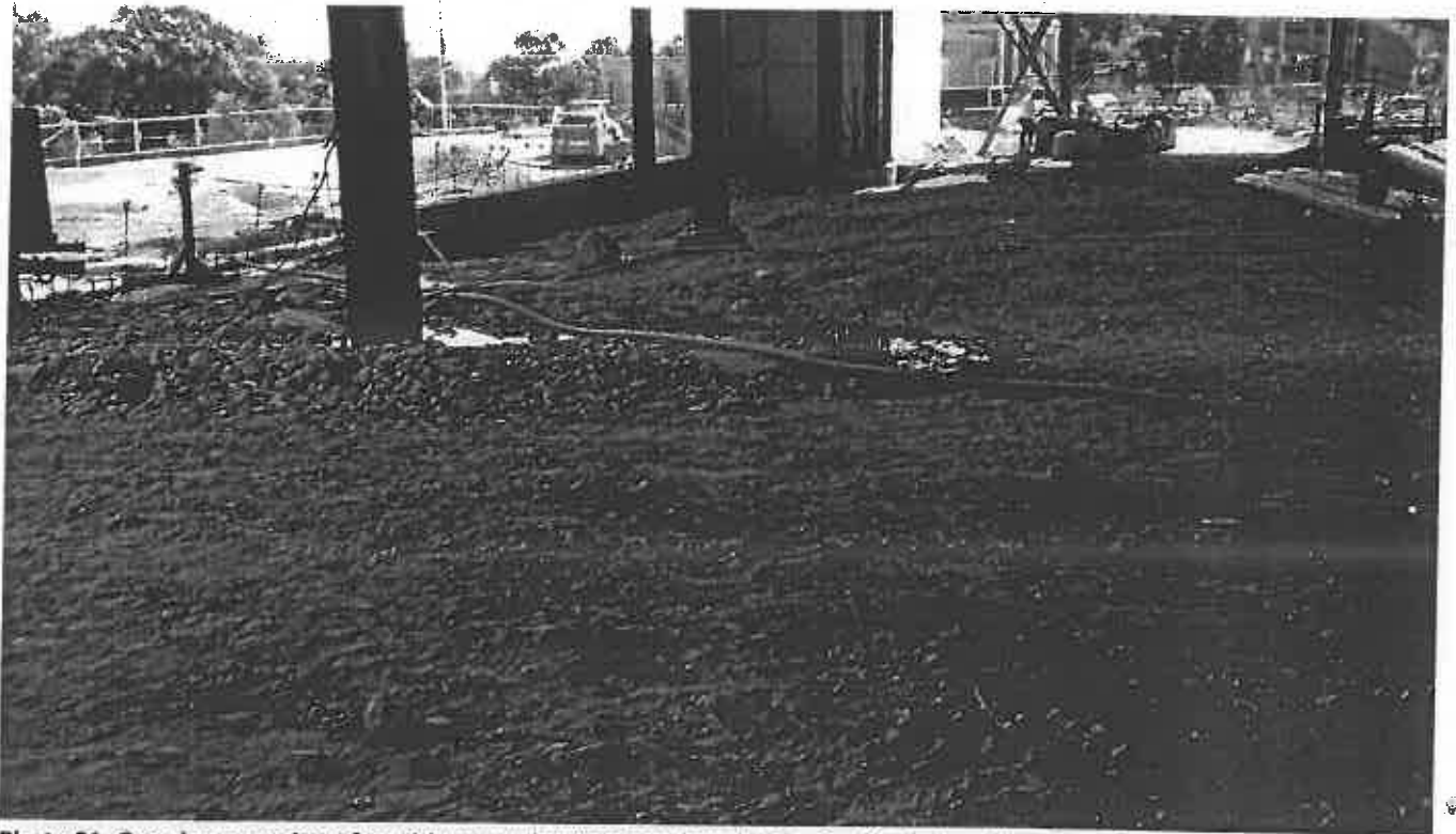
Photo 21. Ongoing pumping of muddy groundwater from foundation footing into active stormdrain onsite.
