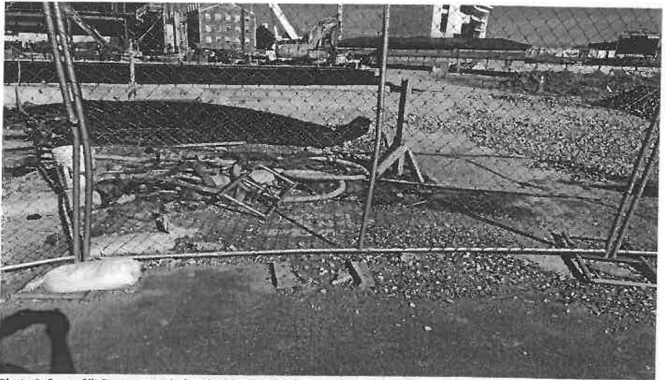
Photo 1. Super Silt Fence overwhelmed with pile of sediment North of the site
