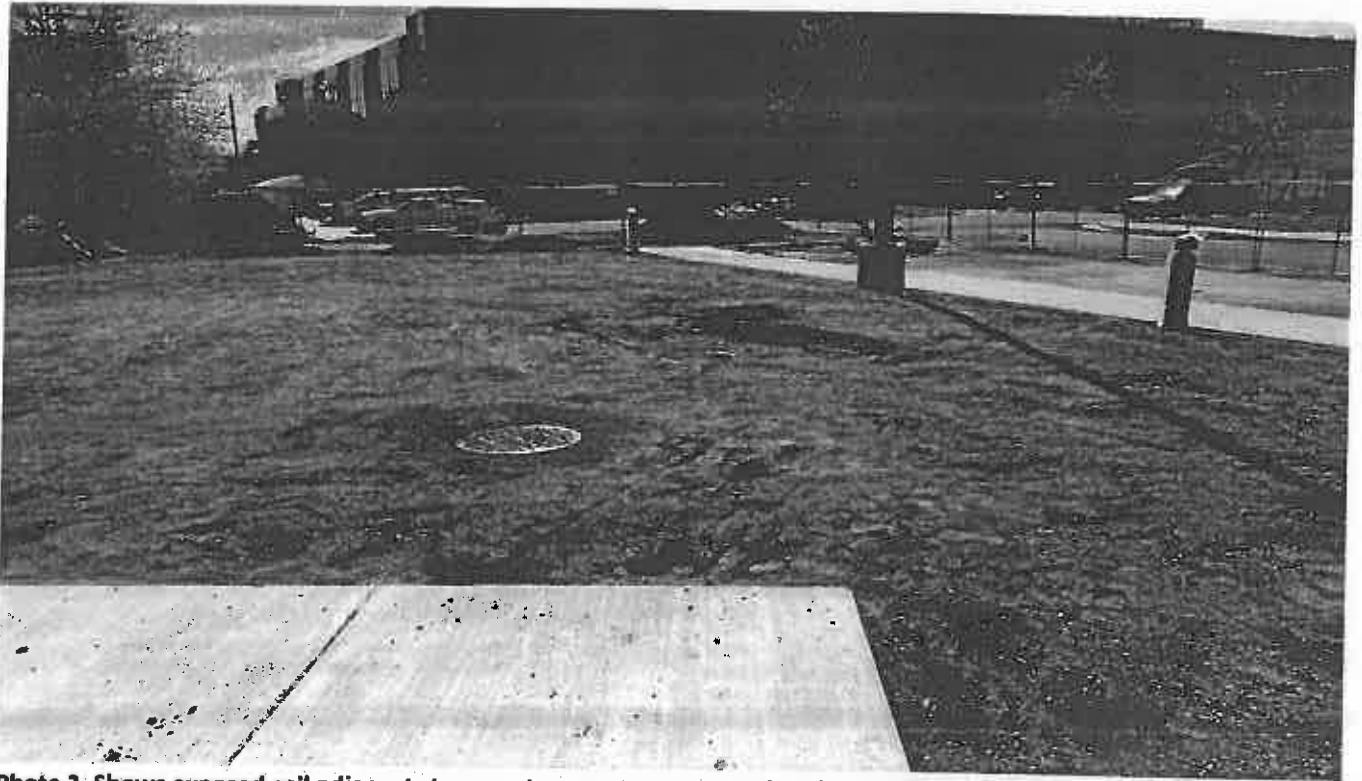
Photo 2. Shows exposed soil adjacent storm water management pond at the new tennis court
