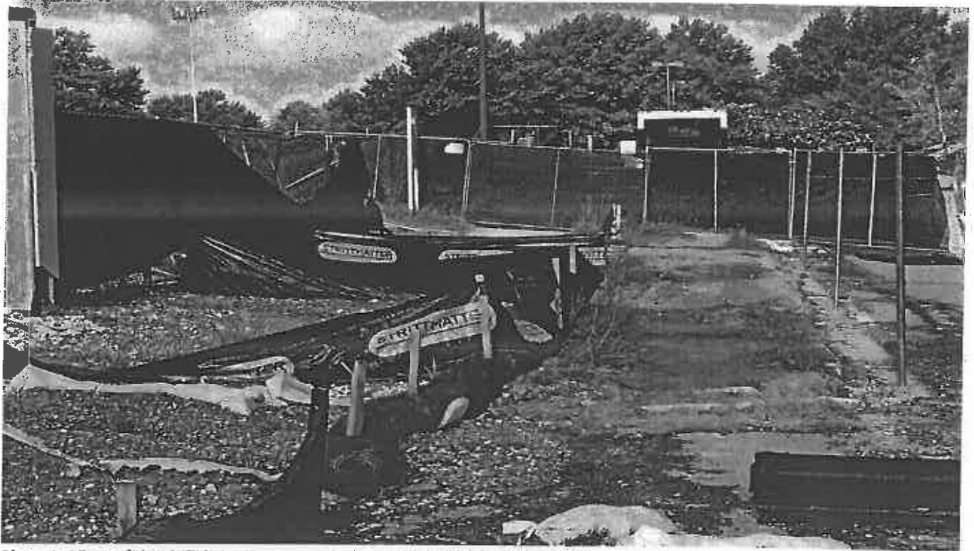
Photo 7. View of the deficient erosion and sediment control SW of the site
