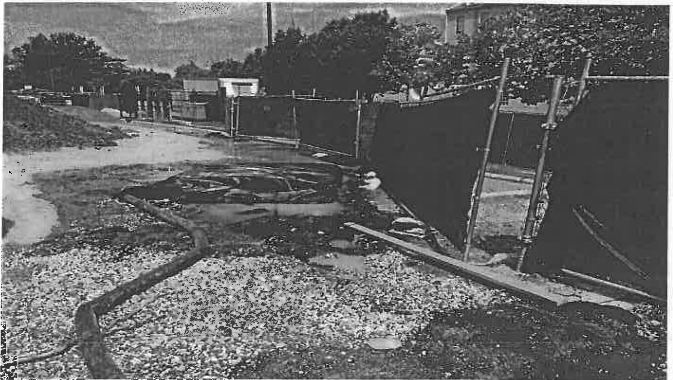
Photo 4. Sediment filter bag placed on exposed soil NW of the site near the sediment tank going into stormdrain
