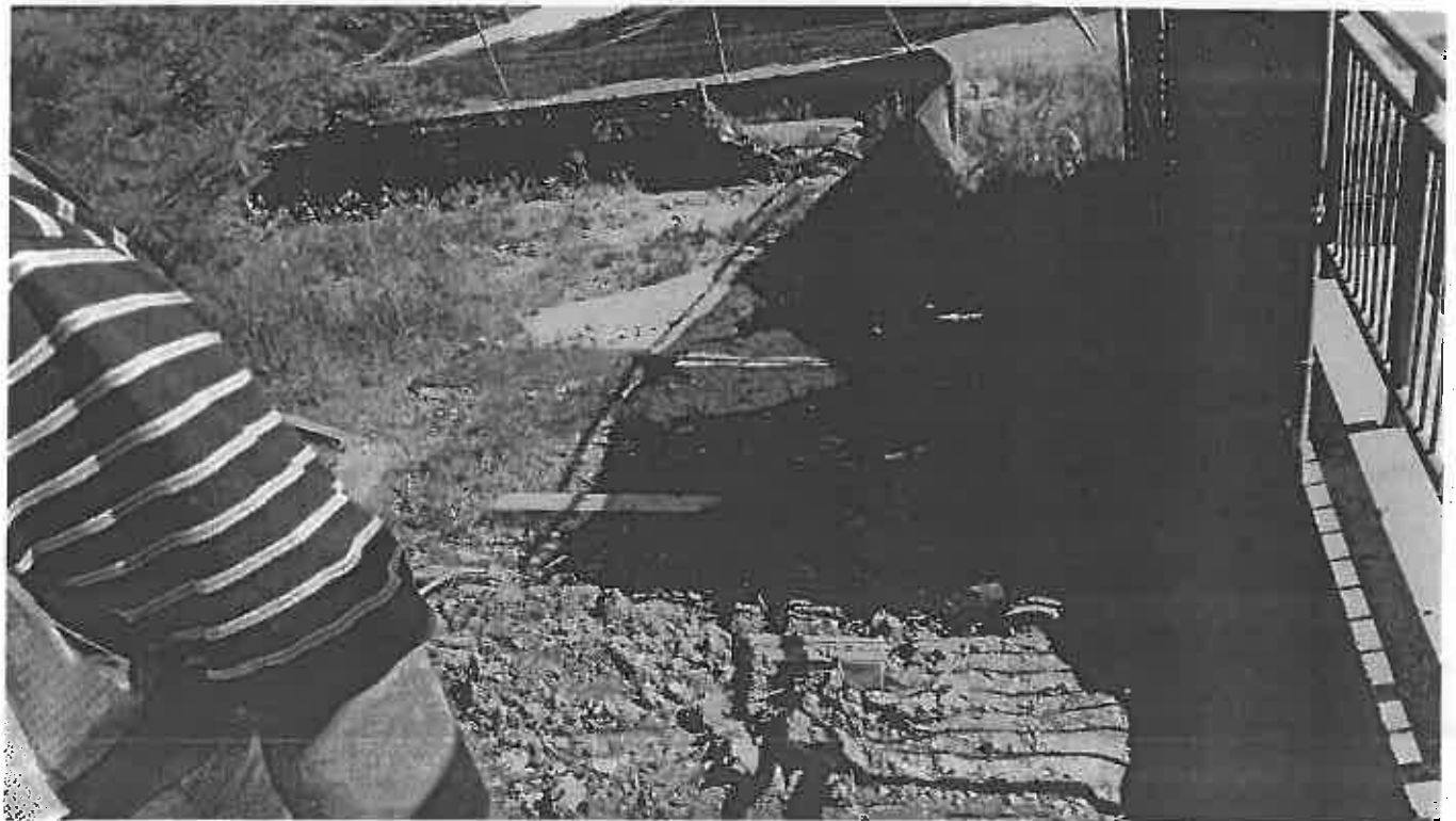
Photo 4. Unmaintained E and S controls at the Slope of the Tunnel Project North of the Site
