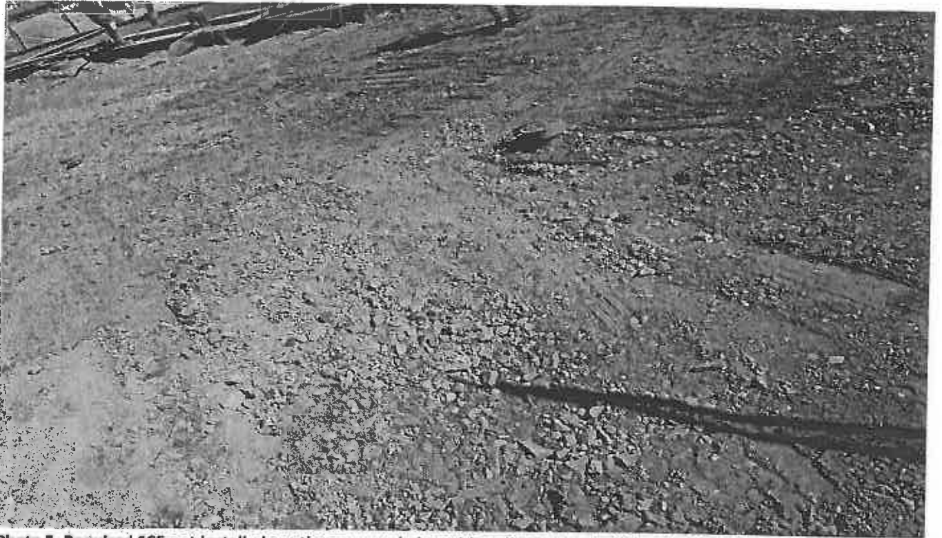
Photo 5. Required SCE not installed per the approved plan with sediment track off the site NE of the side.
