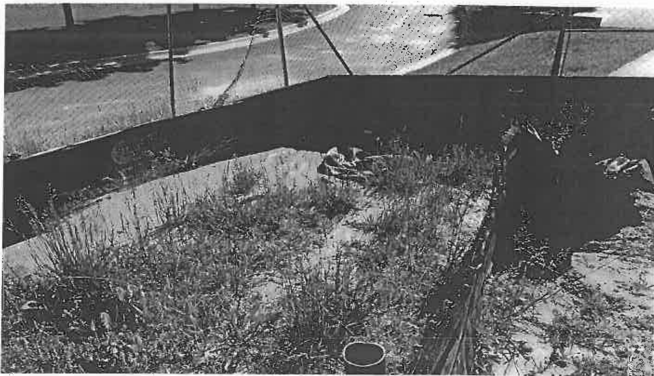
Photo 2. Accumulated silt and sediment at the E and S control footings at the Slope of the Tunnel Project North of the Site
