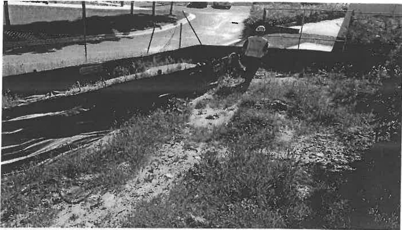
Photo 1. SSF not properly trenched to the ground at the Slope of the Tunnel Project North of the Site
