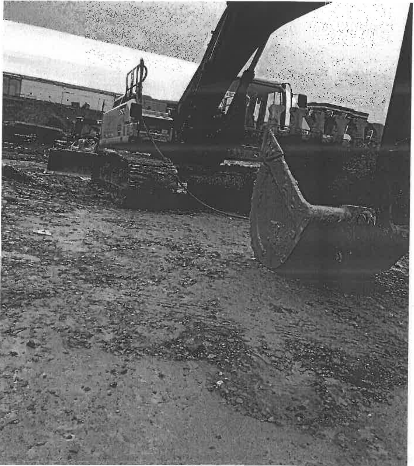
Photo 13. Stabilized Construction Entrance with little or no stones despite ongoing rain event.
