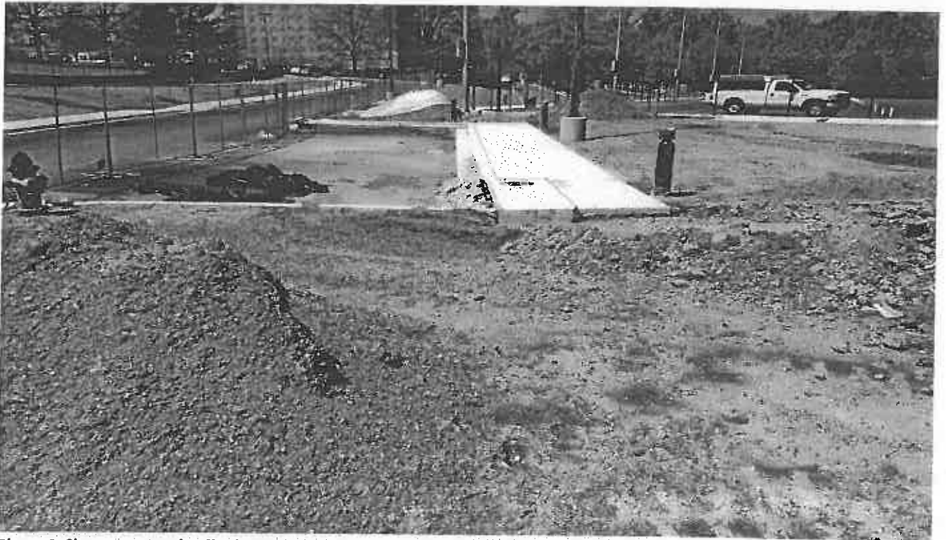
Photo 4. Shows exposed soil adjacent storm water management pond at the new tennis court
