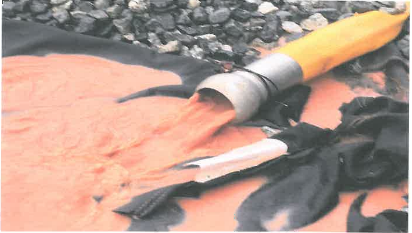
Photo 5. Ongoing pumping of Sediment laden Stormwater into active stormdrain onsite (State Waters)
