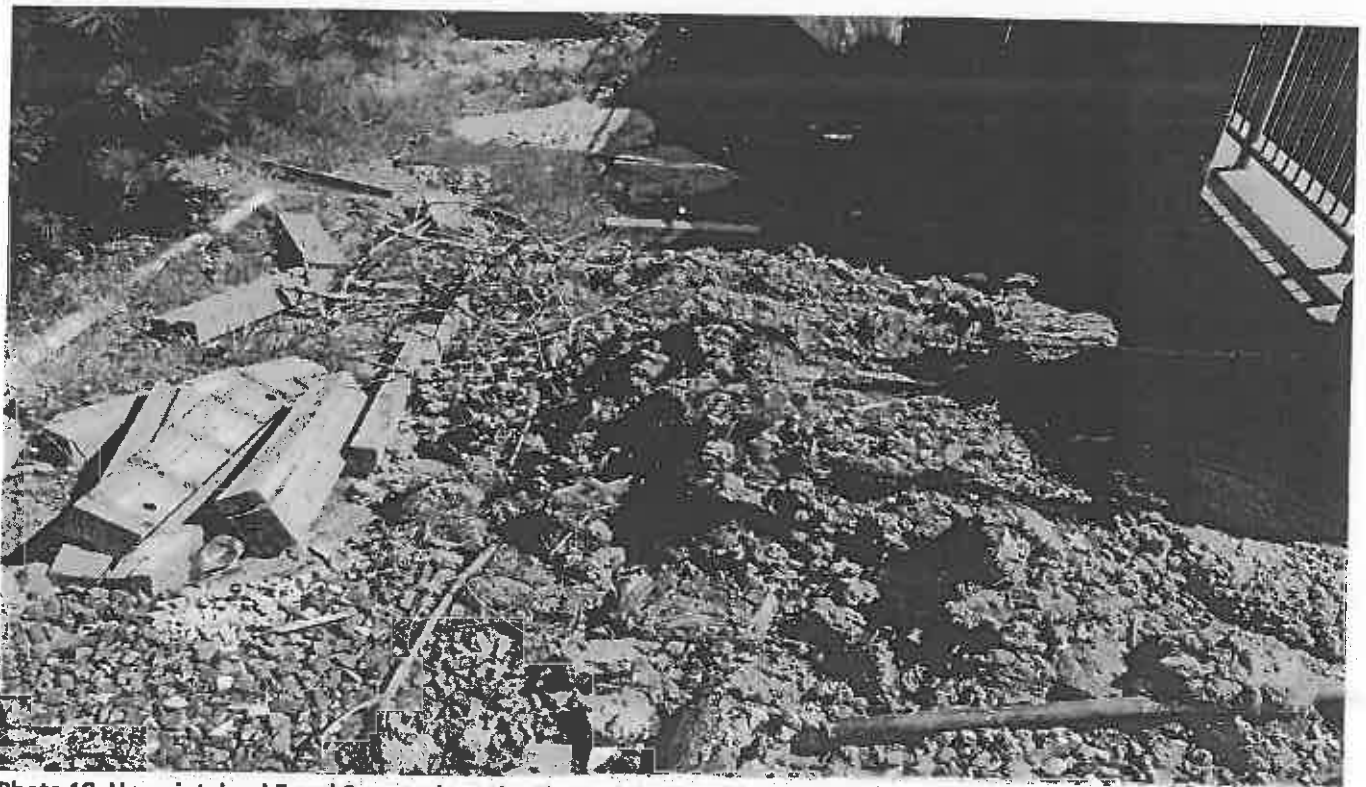
Photo 18. Unmaintained E and S controls at the Slope of the Tunnel Project North of the Site
