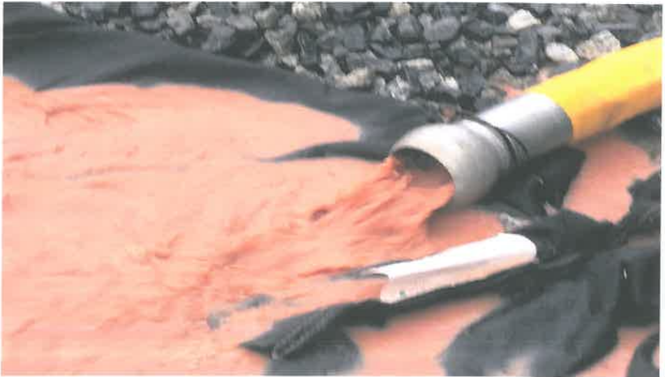
Photo 4. Ongoing pumping of Sediment laden Stormwater into active stormdrain onsite (State Waters)
