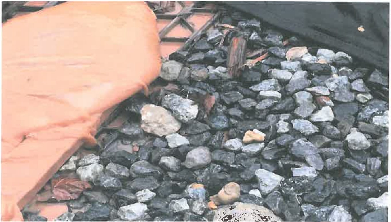
Photo 6. Ongoing pumping of Sediment laden Stormwater into active stormdrain onsite (State Waters)
