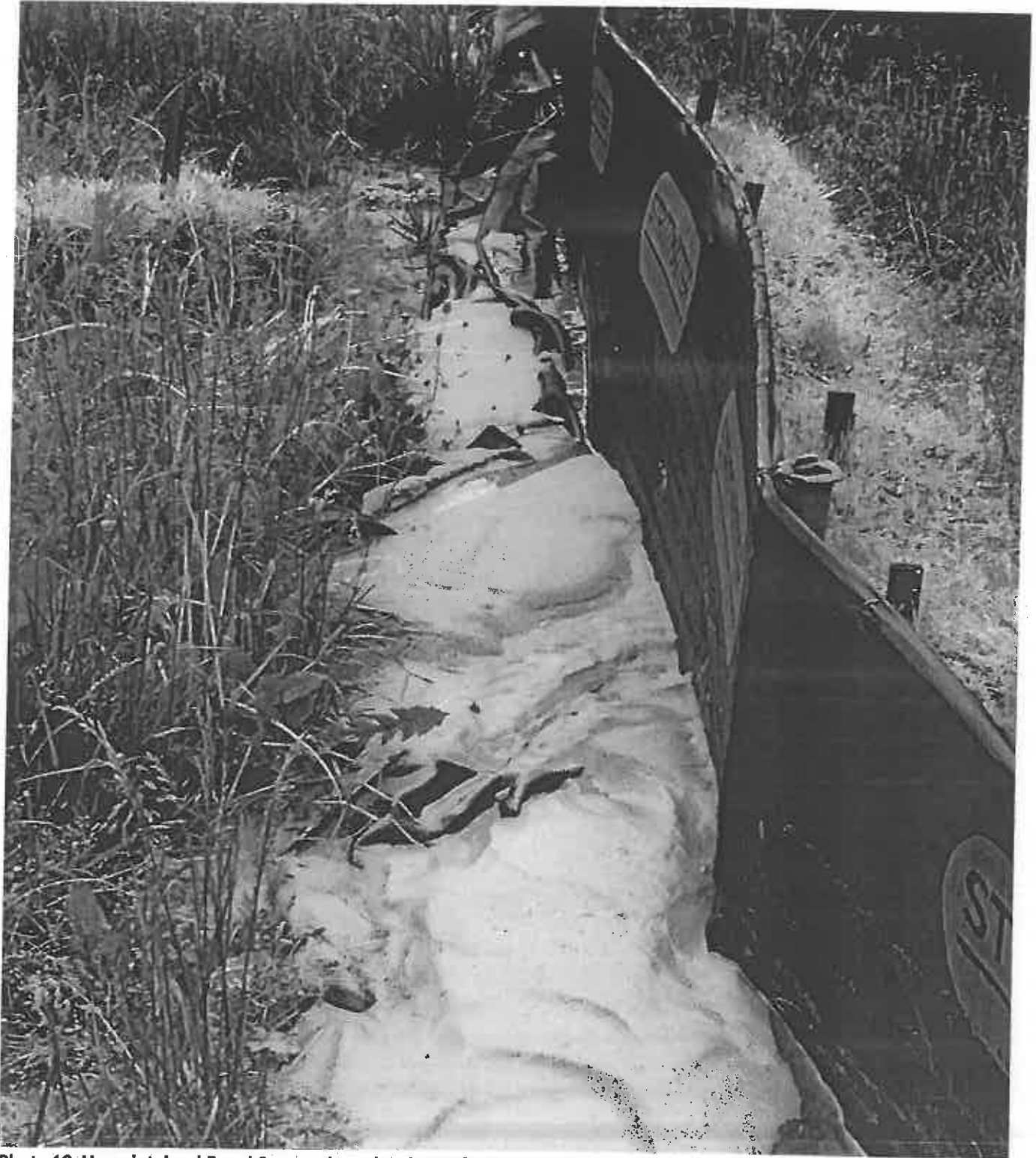
Photo 10. Unmaintained E and S controls at the Slope of the Tunnel Project North of the Site
