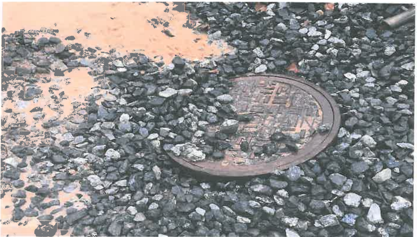
Photo 14. Ongoing pumping of Sediment laden Stormwater into active stormdrain onsite (State Waters)
