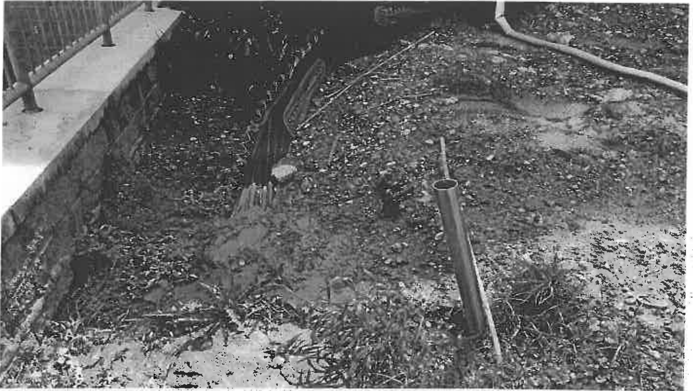
Photo 12. Unmaintained E and S controls at the Slope of the Tunnel Project North of the Site
