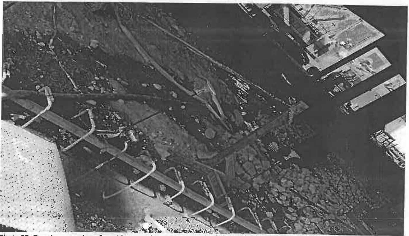
Photo 22. Ongoing pumping of muddy groundwater from foundation footing into active stormdrain onsite.
