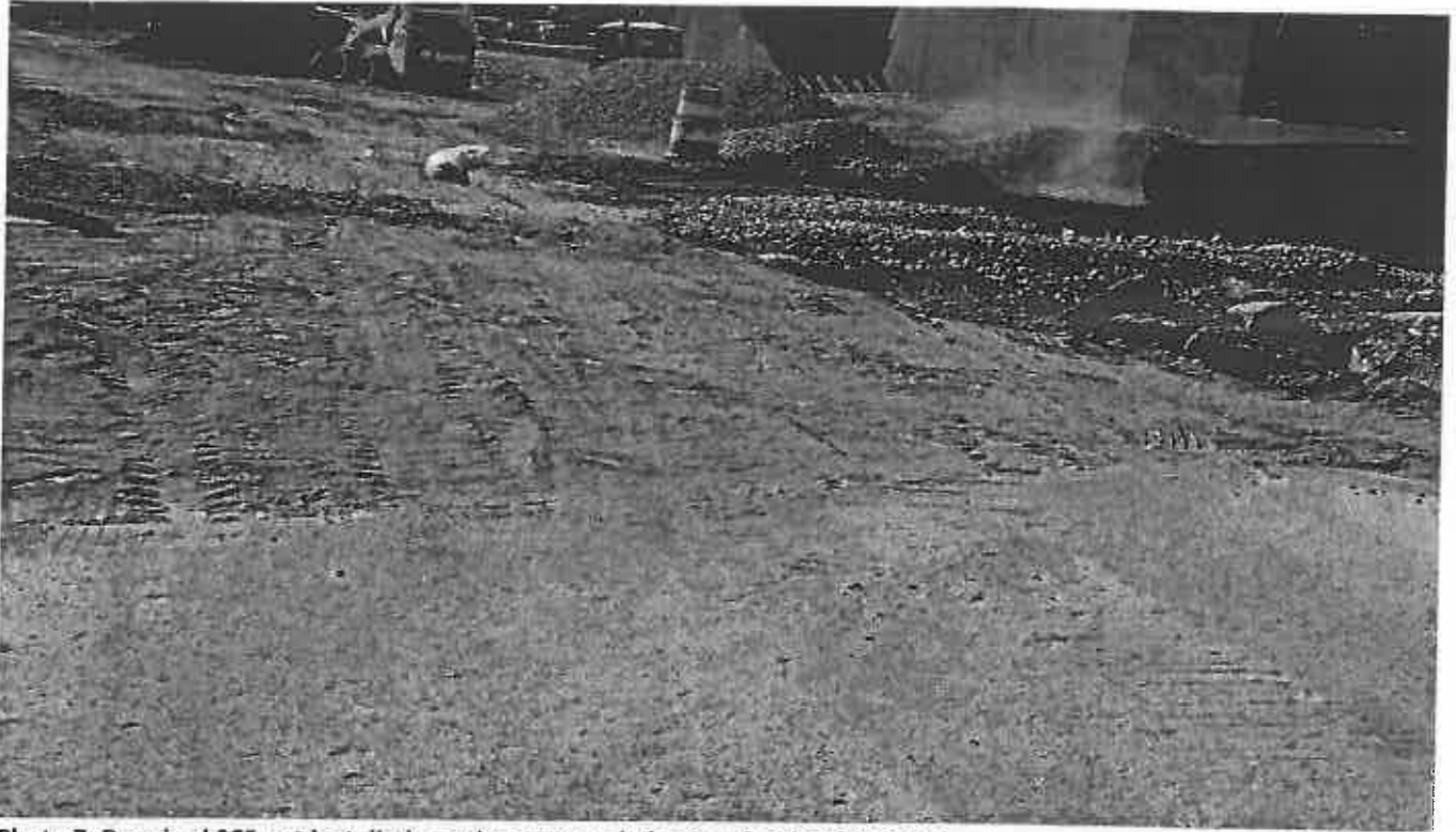
Photo 7. Required SCE not installed per the approved plan South side of the site
