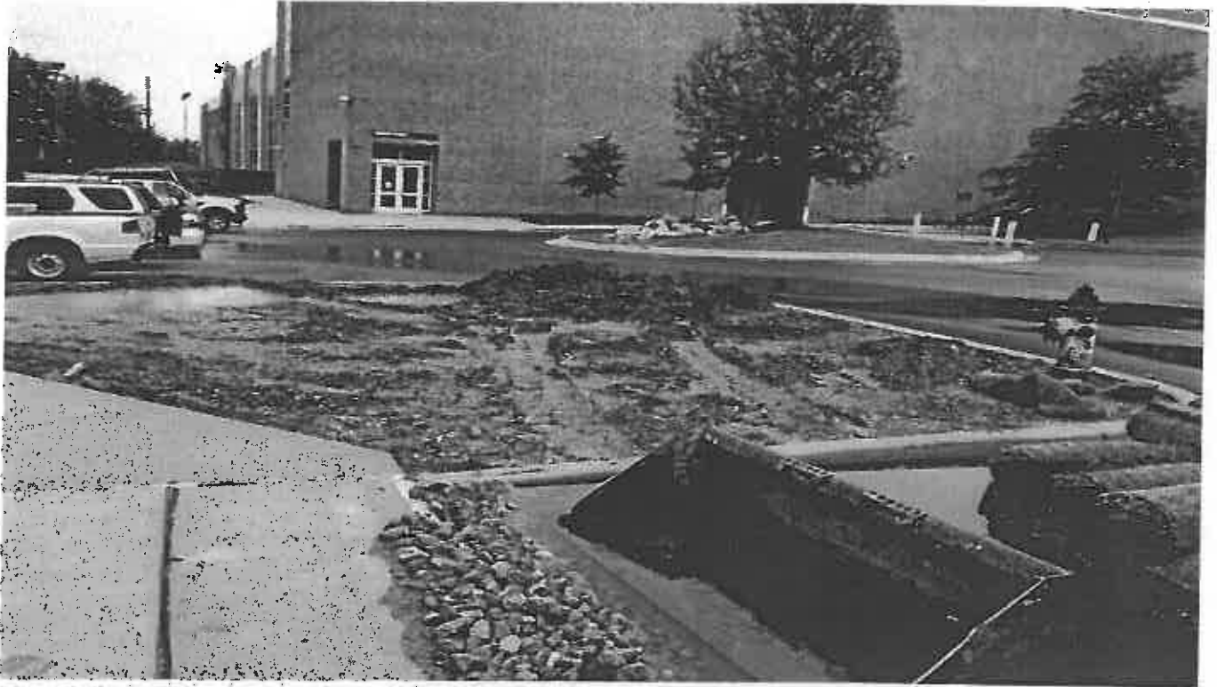
Photo 3. Shows sod and mud at the parking lot adjacent the sport center and the Curb storm Drain
