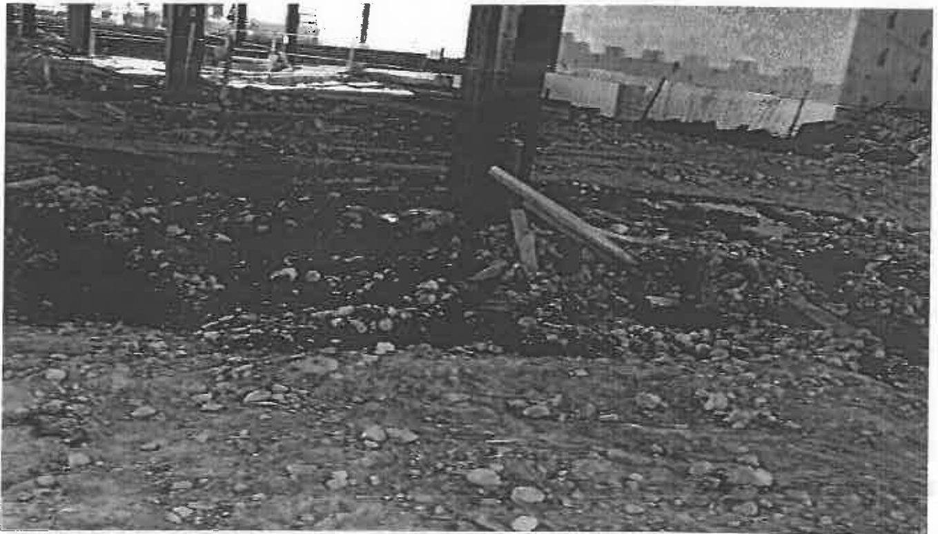
Photo 20. Ongoing pumping of muddy groundwater from foundation footing into active stormdrain onsite.
