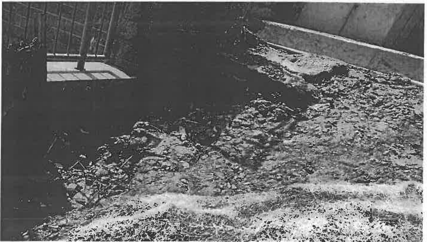
Photo 13. Unmaintained E and S controls at the Slope of the Tunnel Project North of the Site
