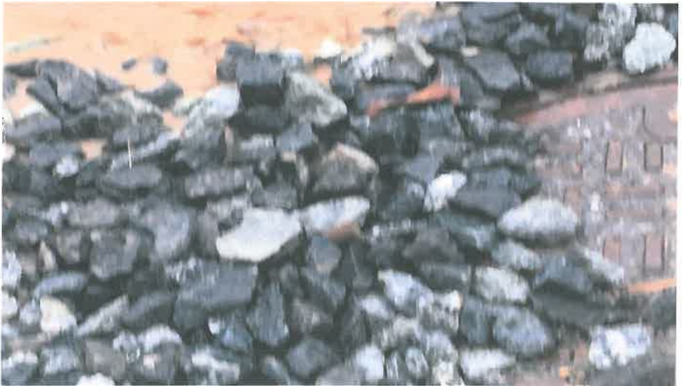
Photo 12. Ongoing pumping of Sediment laden Stormwater into active stormdrain onsite (State Waters)
