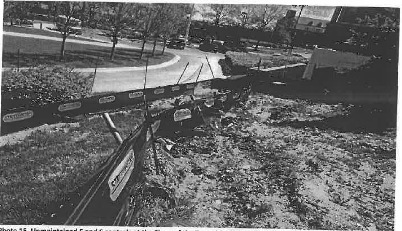
Photo 15. Unmaintained E and S controls at the Slope of the Tunnel Project North of the Site
