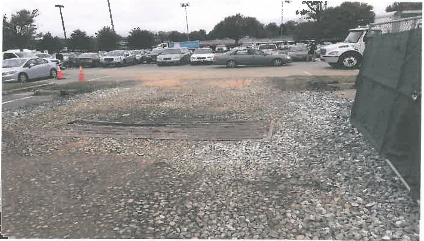
Photo 7. Sediment laden Stabilized Construction Entrance 2 Exit to the Car Park
