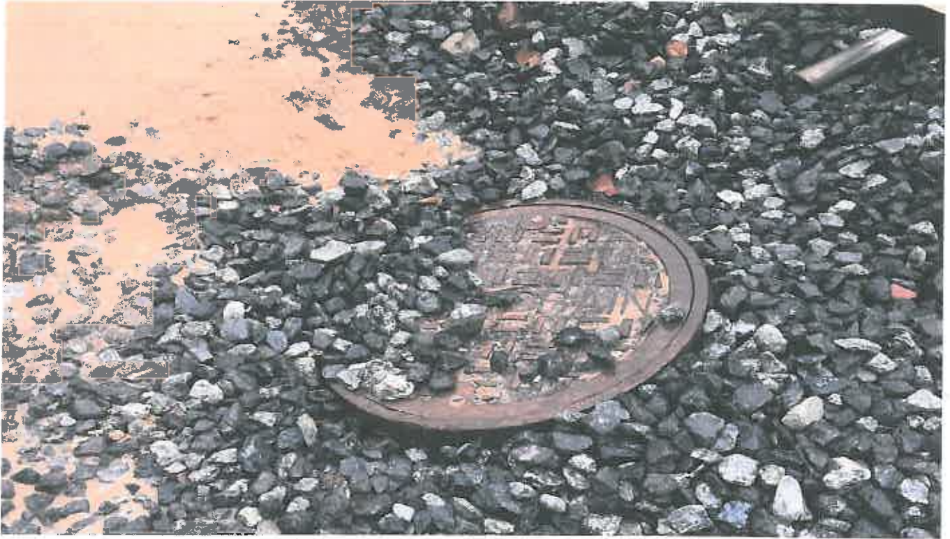
Photo 13. Ongoing pumping of Sediment laden Stormwater into active stormdrain onsite (State Waters)
