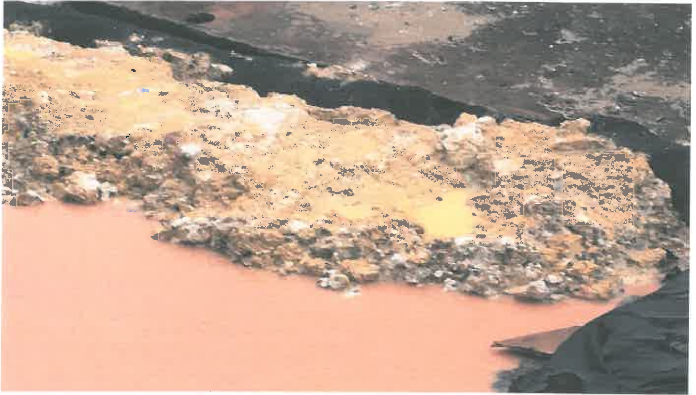
Photo 9. Ongoing pumping of Sediment laden Stormwater into active stormdrain onsite (State Waters)
