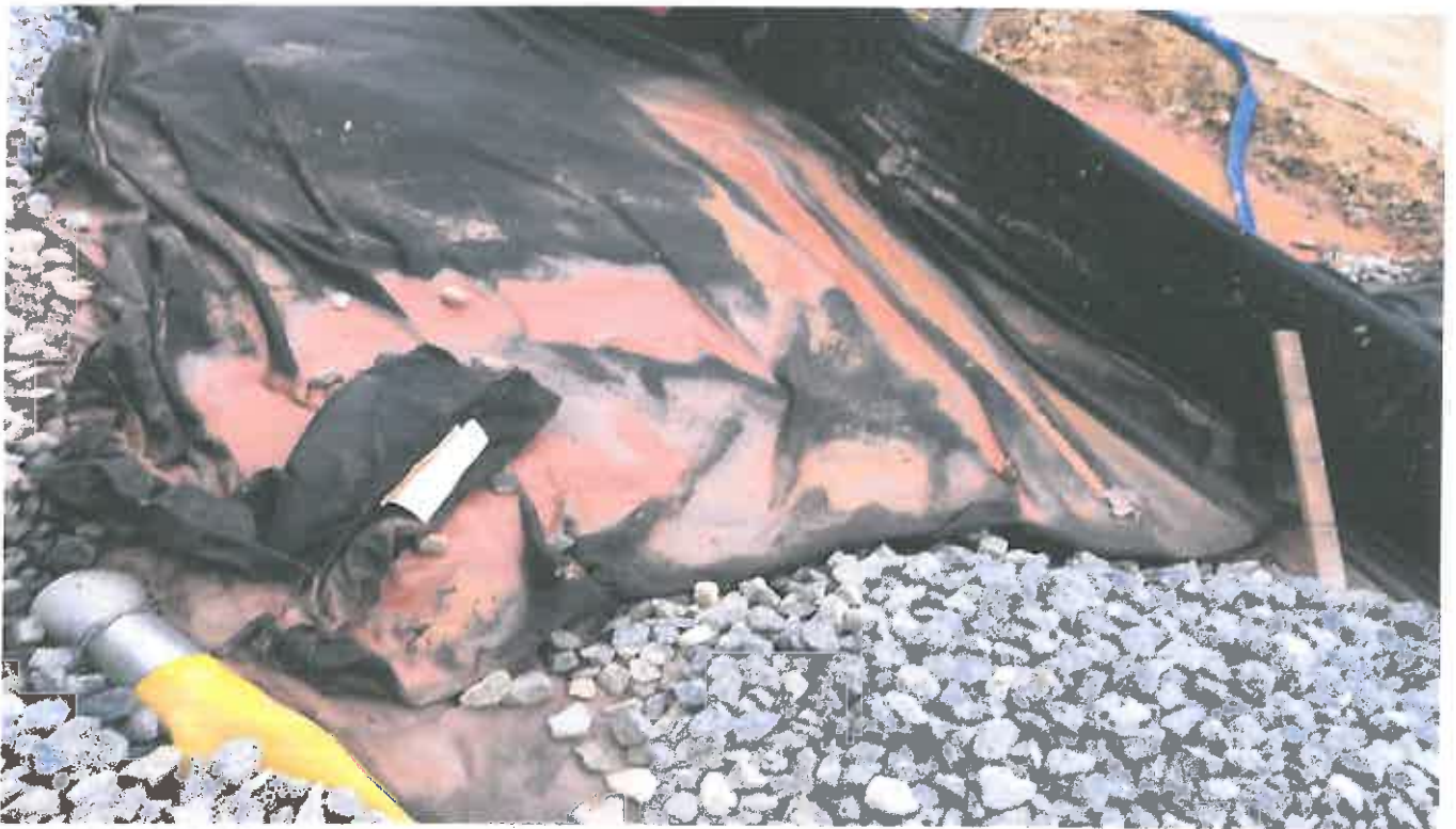
Photo 4. Muddy Silt Bag or Filter Bag with Close Proximity to the Stormdrain
