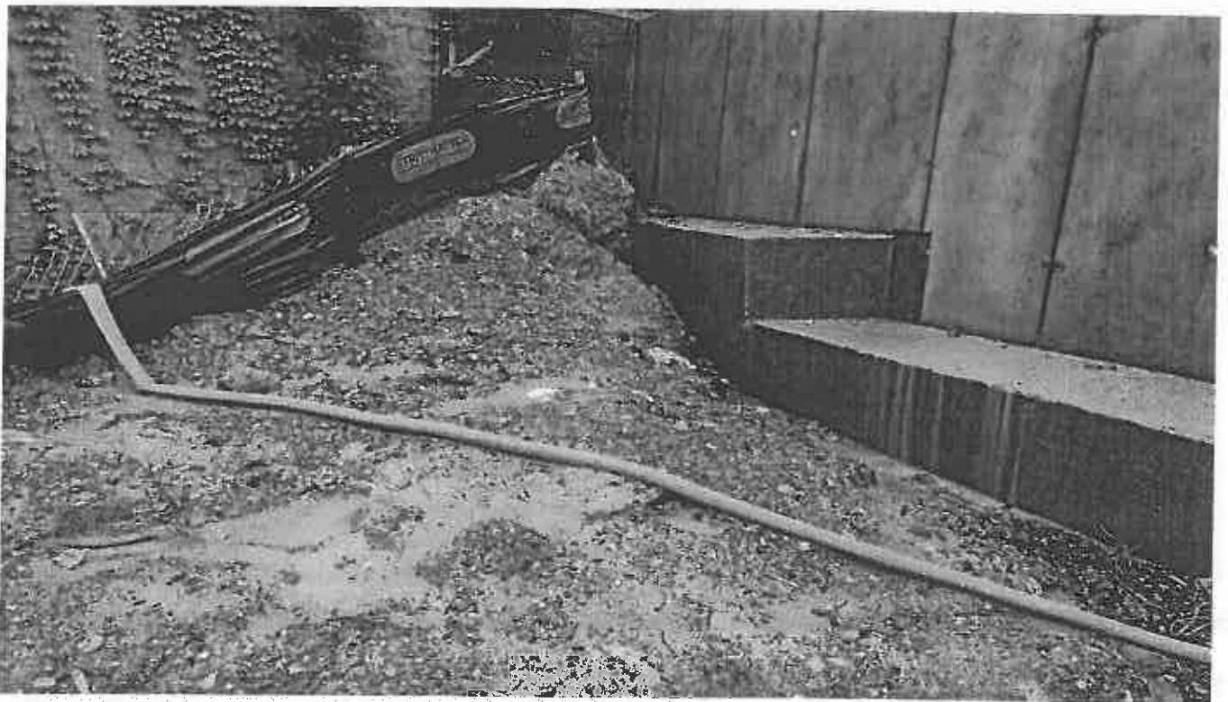
Photo 6. Unmaintained E and S controls at the Slope of the Tunnel Project North of the Site
