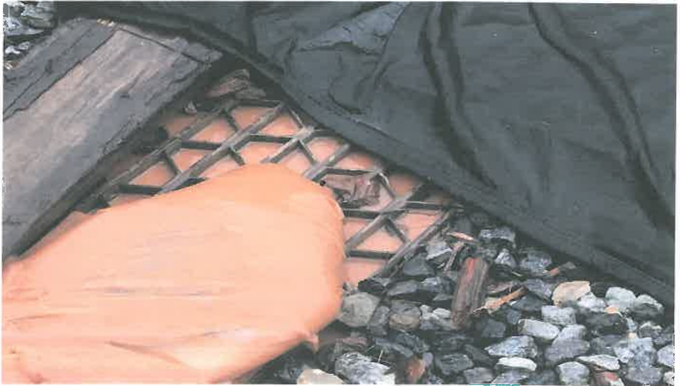
Photo 8. Ongoing pumping of Sediment laden Stormwater into active stormdrain onsite (State Waters)
