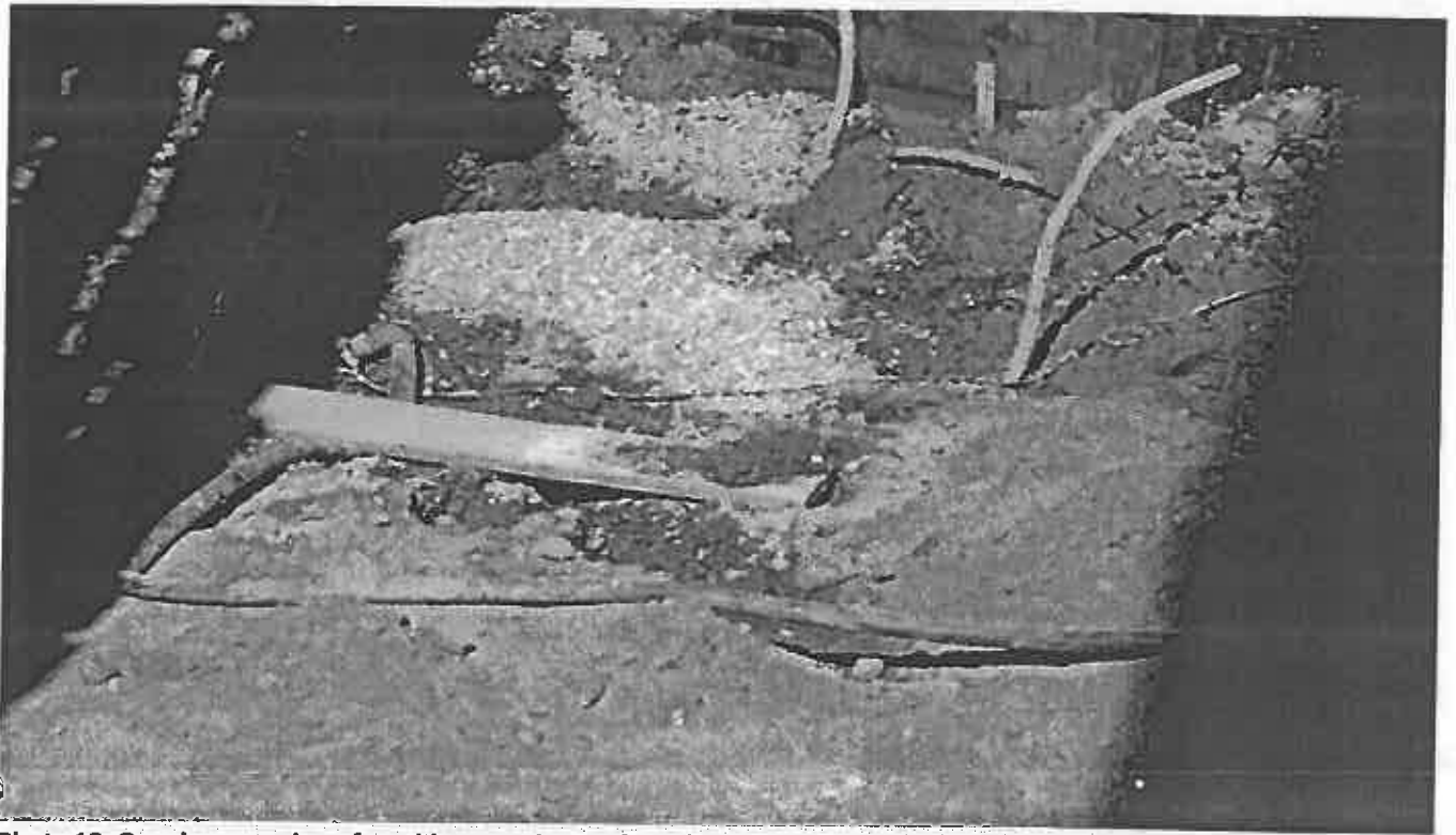
Photo 12. Ongoing pumping of muddy groundwater from foundation footing into active stormdrain onsite.
