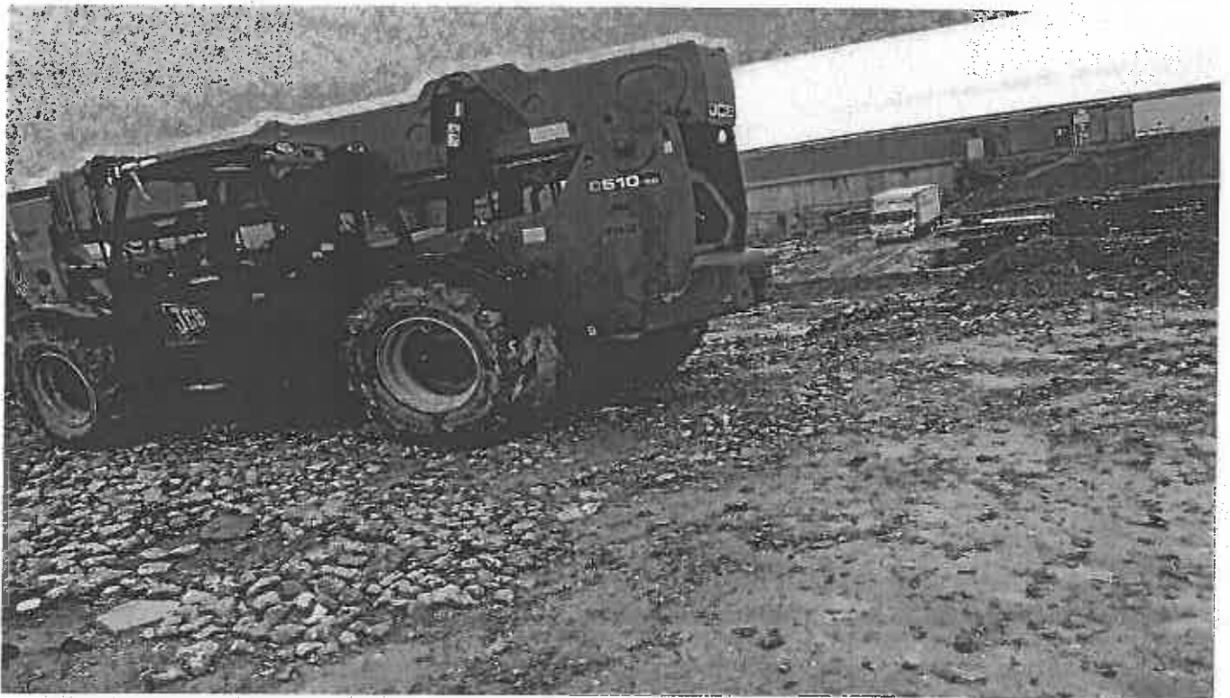
Photo 12. Stabilized Construction Entrance with little or no stones despite ongoing rain event.
