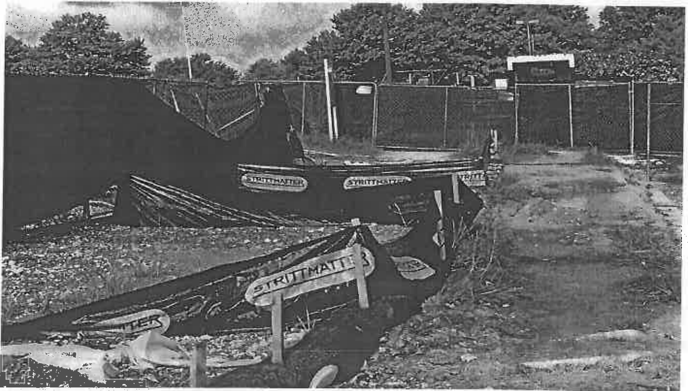
Photo 8. View of the deficient erosion and sediment control SW of the site
