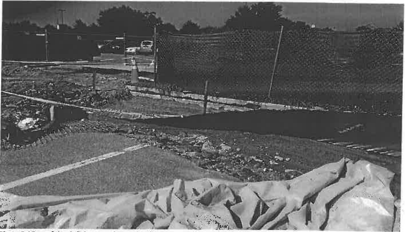
Photo 9. View of the deficient erosion and sediment control South of the site
