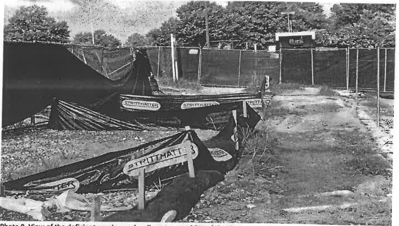
Photo 9. View of the deficient erosion and sediment control SW of the site
