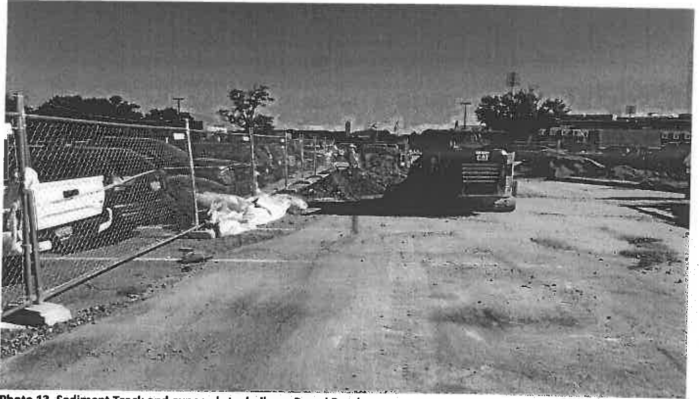
Photo 13. Sediment Track and exposed stockpile on Paved Road
