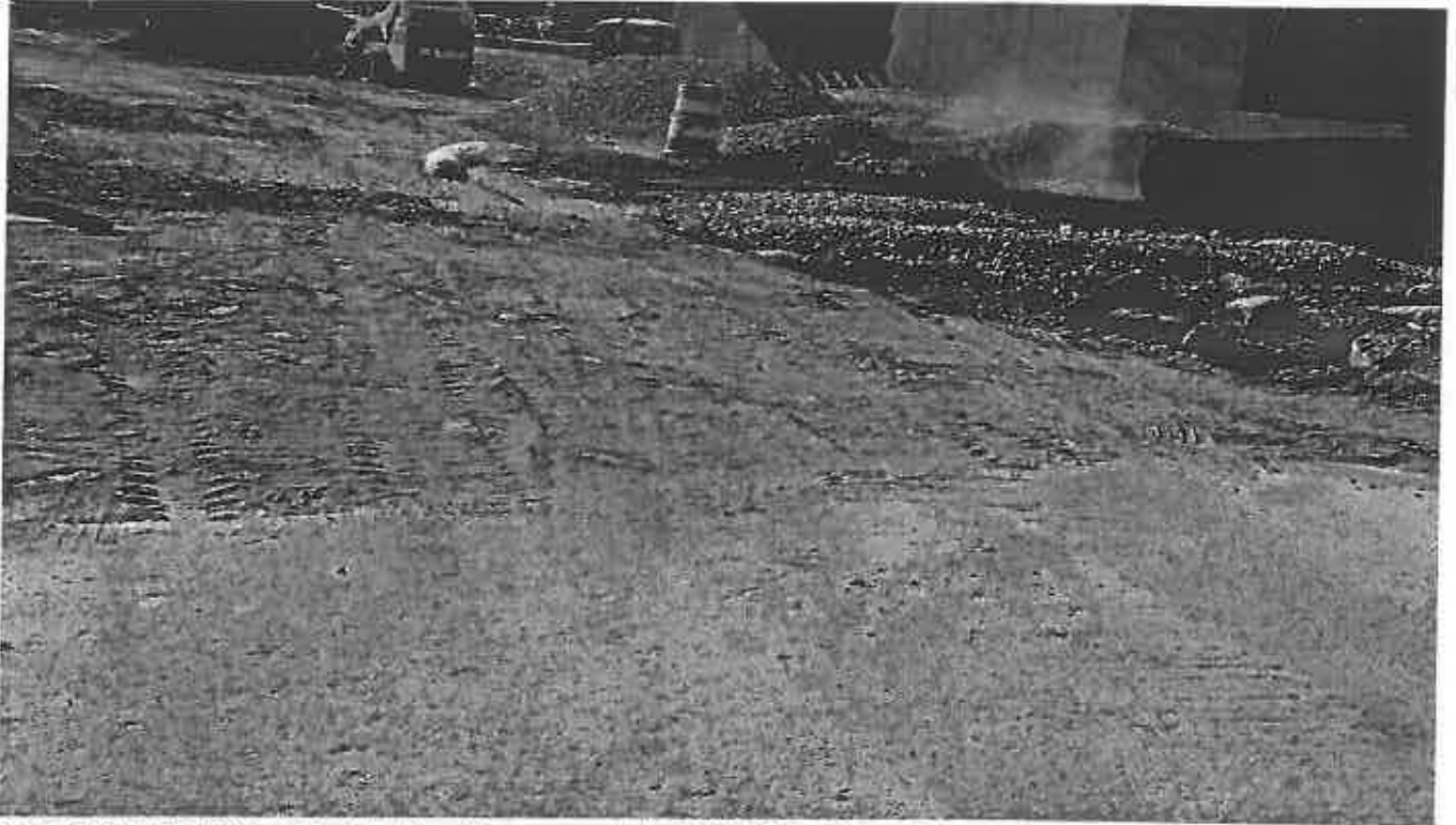
Photo 5. Required SCE not installed per the approved plan NW of the site.
