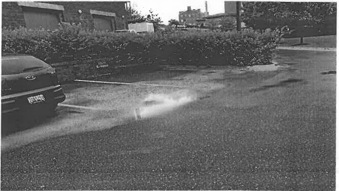
Photo 12. Sediment laden stormwater runoff from site to the stormdrain at Gossett Football Team House lot.
