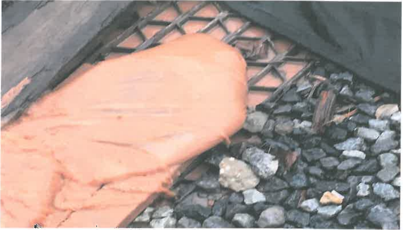
Photo 7. Ongoing pumping of Sediment laden Stormwater into active stormdrain onsite (State Waters)
