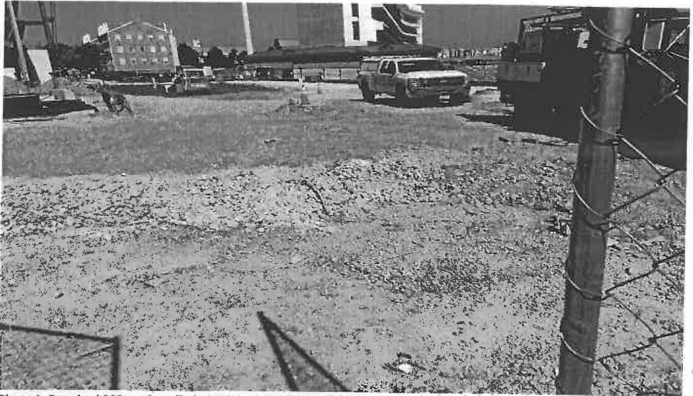
Photo 1. Required SCE not installed per the approved plan NE of the site.
