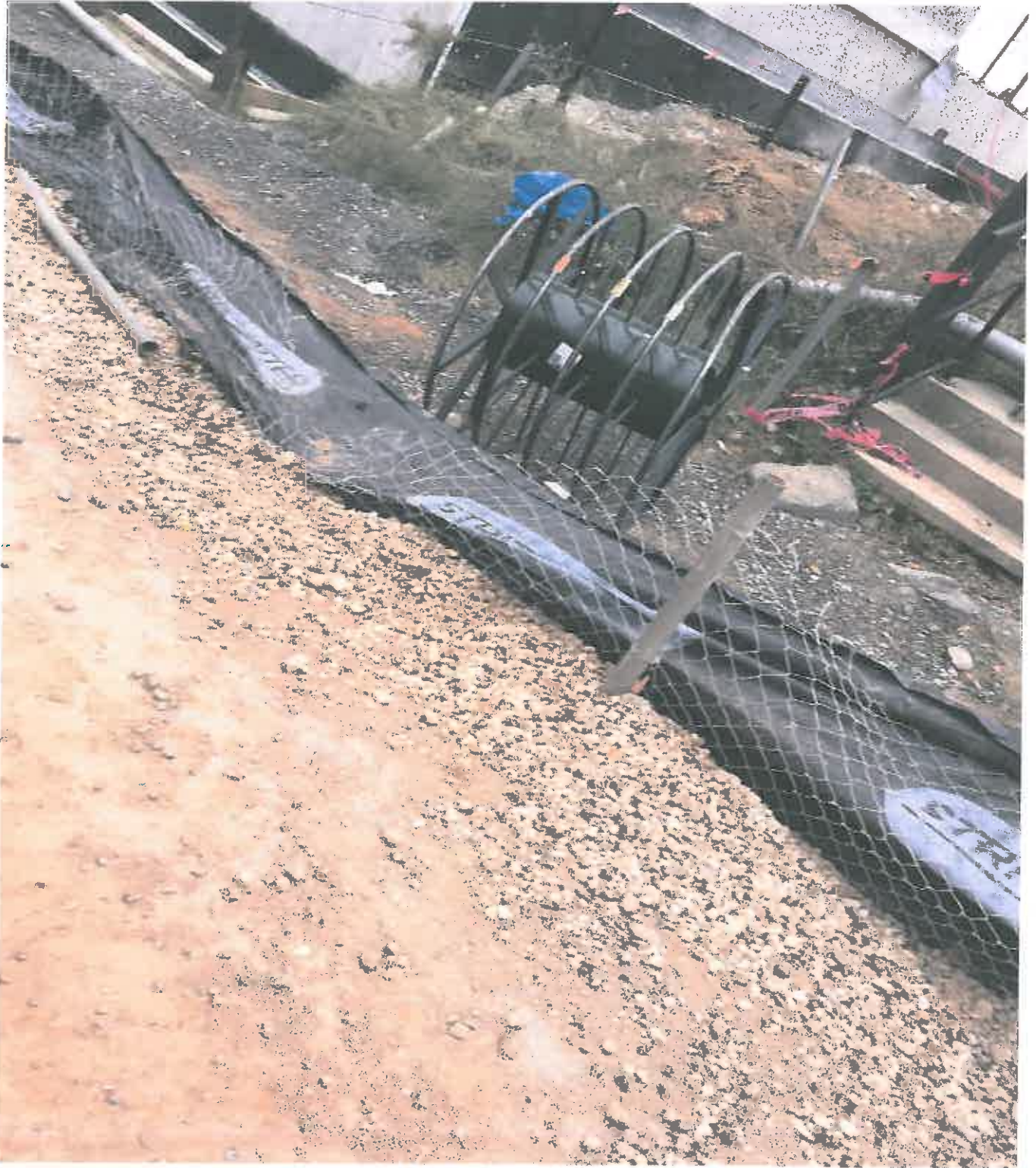
Photo 1. Shows Unmaintained and Compromised Super Silt Fence (SSF) off Cole Field House Drive
