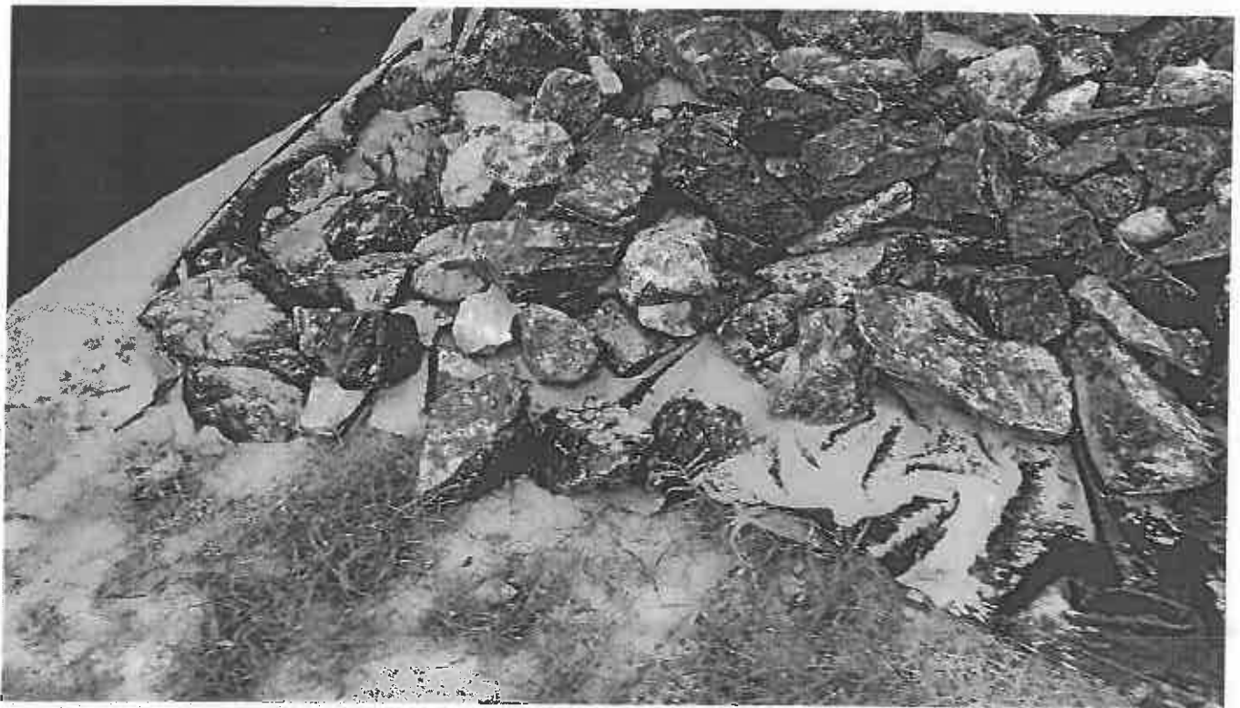
Photo 10. Accumulated silt and sediment at the E and S control footings at the Slope of the Tunnel Project
