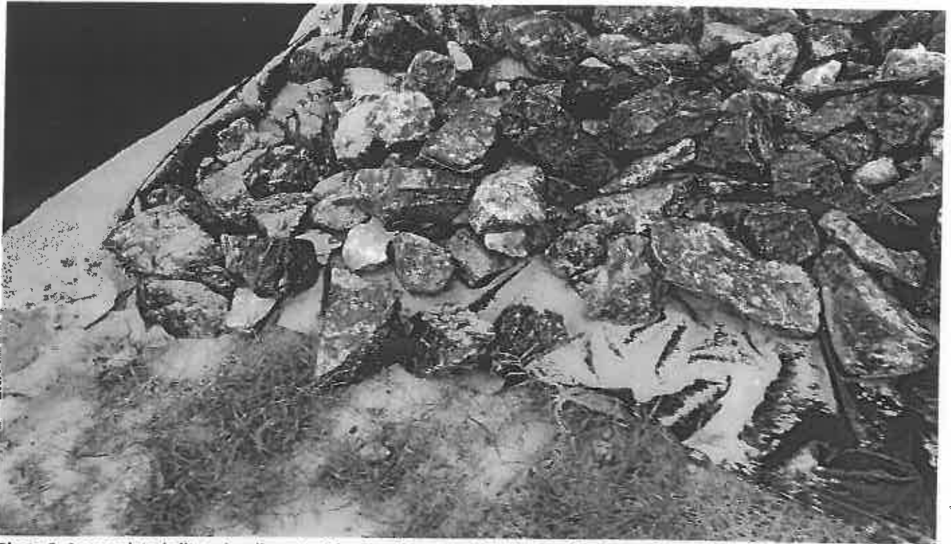
Photo 9. Accumulated silt and sediment at the E and S control footings at the Slope of the Tunnel Project
