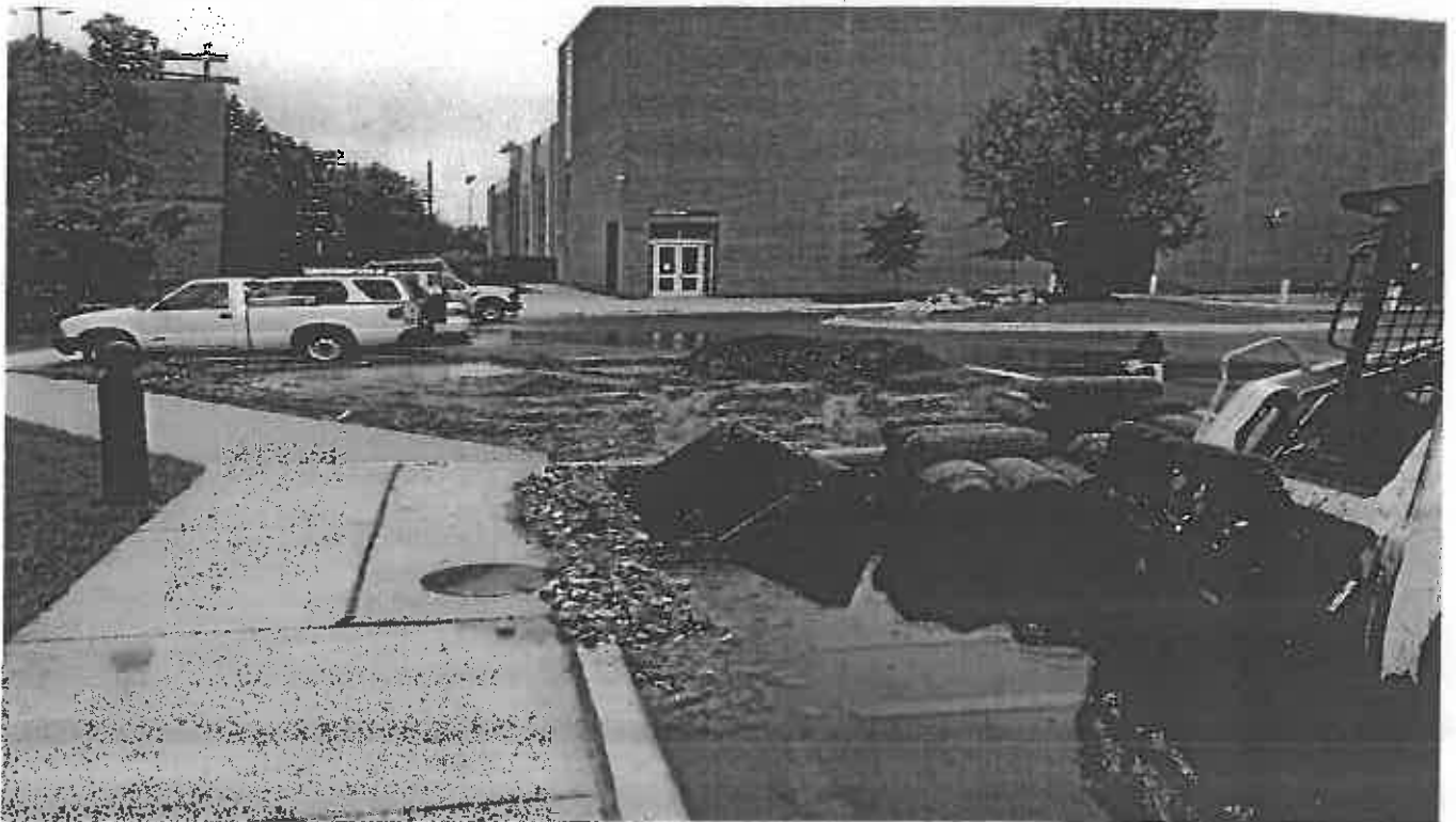
Photo 2. Shows sod and mud at the parking lot adjacent the sport center and the Curb Storm Drain
