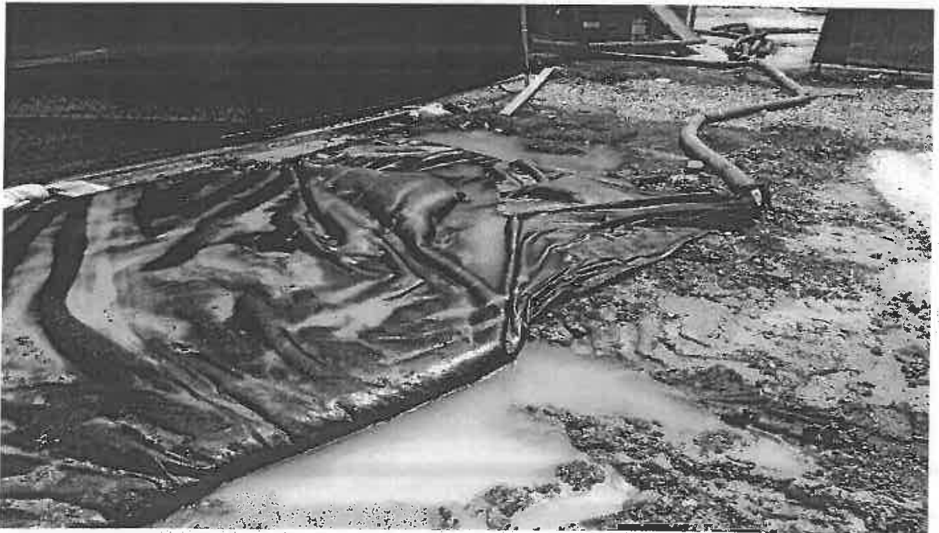
Photo 2. Sediment filter bag placed on exposed soil NW of the site near the sediment tank going into stormdrain
