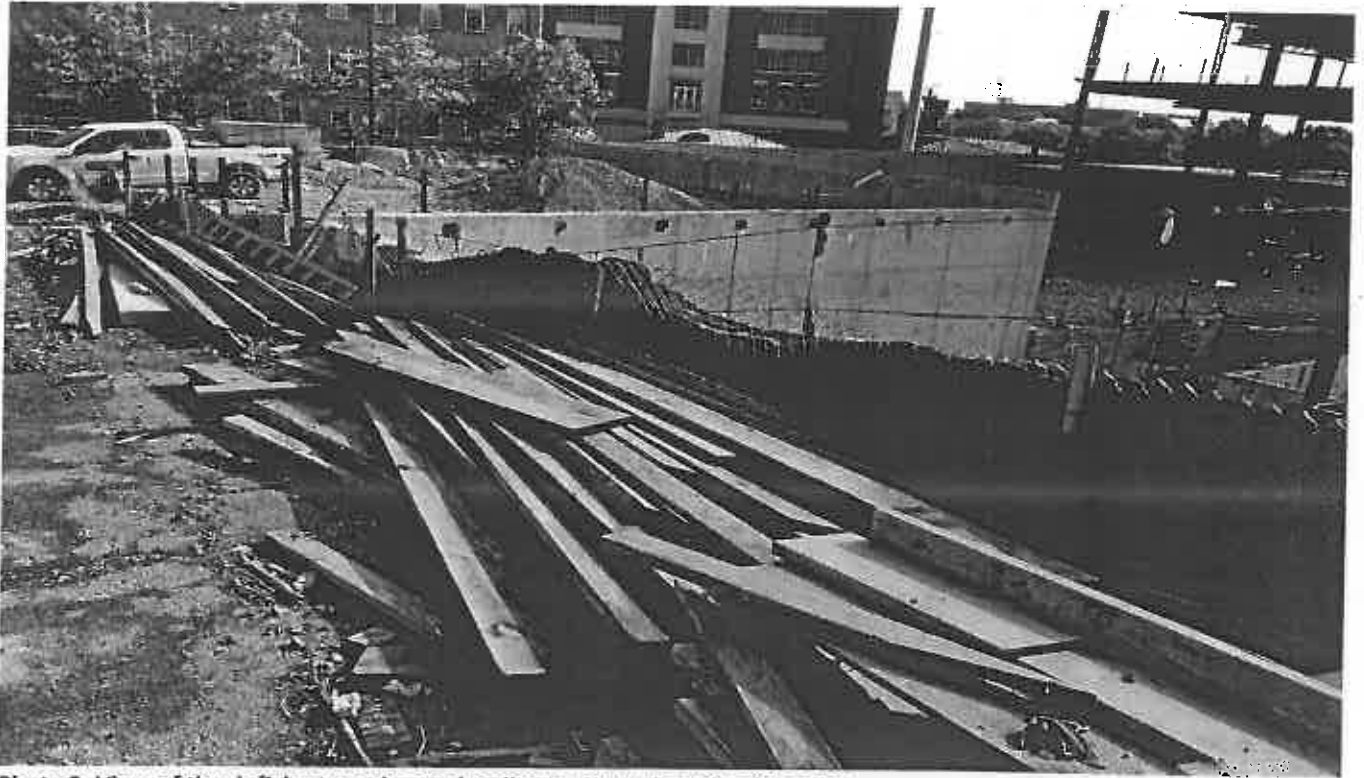
Photo 3. View of the deficient erosion and sediment control South of the site
