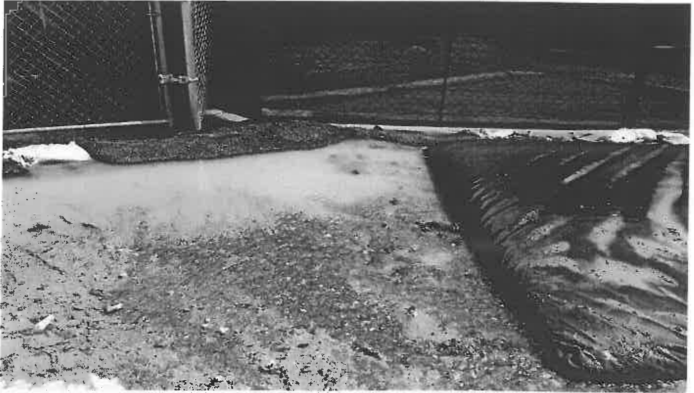
Photo 3. Sediment filter bag placed on exposed soil NW of the site near the sediment tank going into stormdrain
