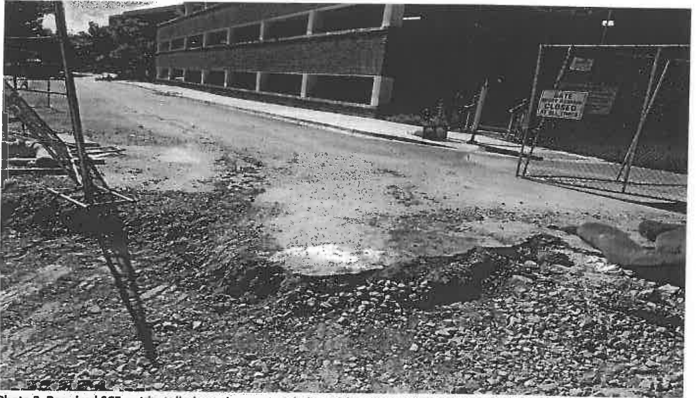
Photo 3. Required SCE not installed per the approved plan with sediment track off the site NE of the side.
