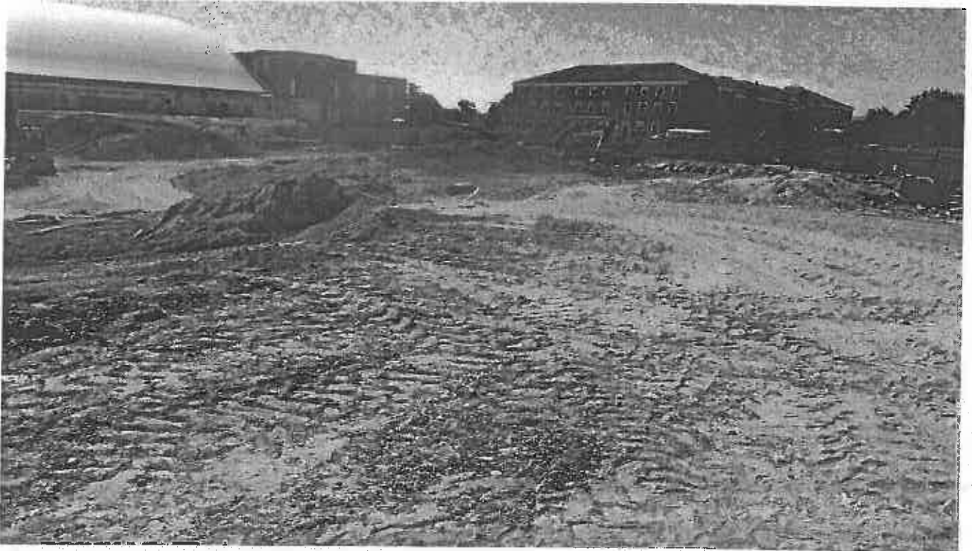
Photo 4. Stabilize Construction Entrance without aggregate stones tracking mud on paved road SW site of site
