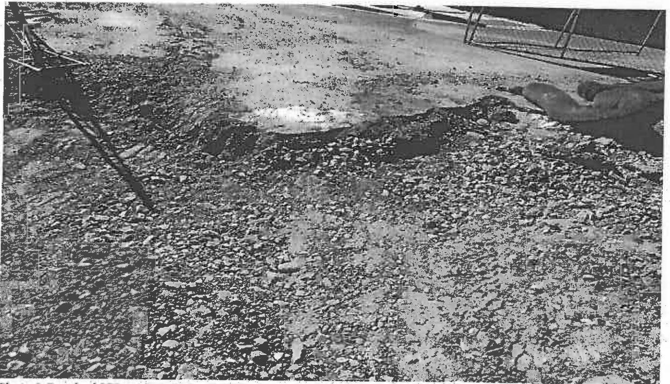
Photo 4. Required SCE not installed per the approved plan with sediment track off the site NE of the side.
