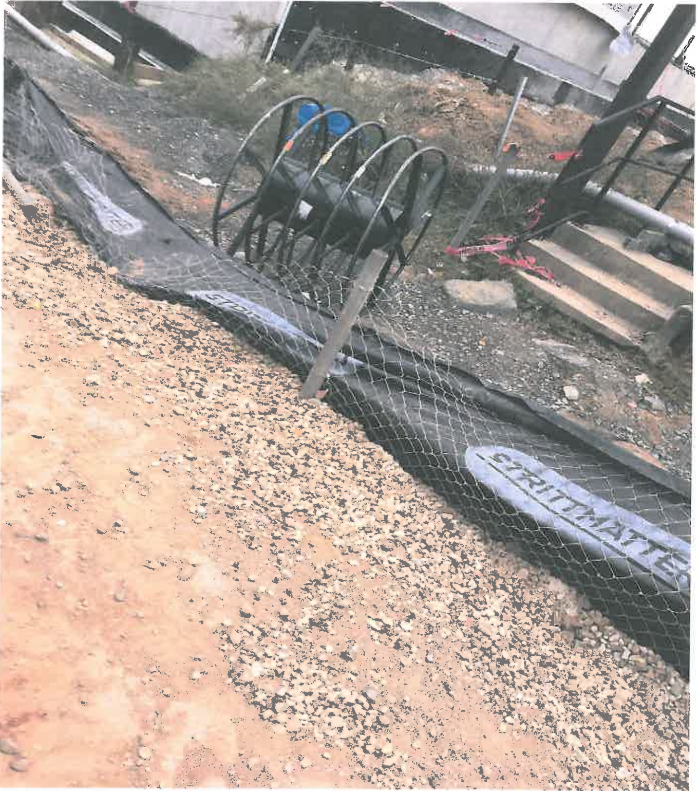
Photo 2. Shows Unmaintained and Compromised Super Silt Fence (SSF) off Cole Field House Drive
