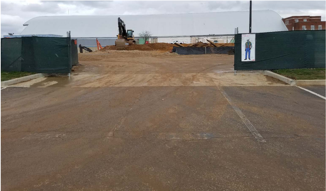
Top: Looking east from Lot Z, major sediment drag-out from the construction site.
