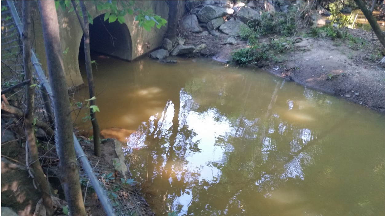
Outfall 005 discharging highly turbid, sediment laden water.
