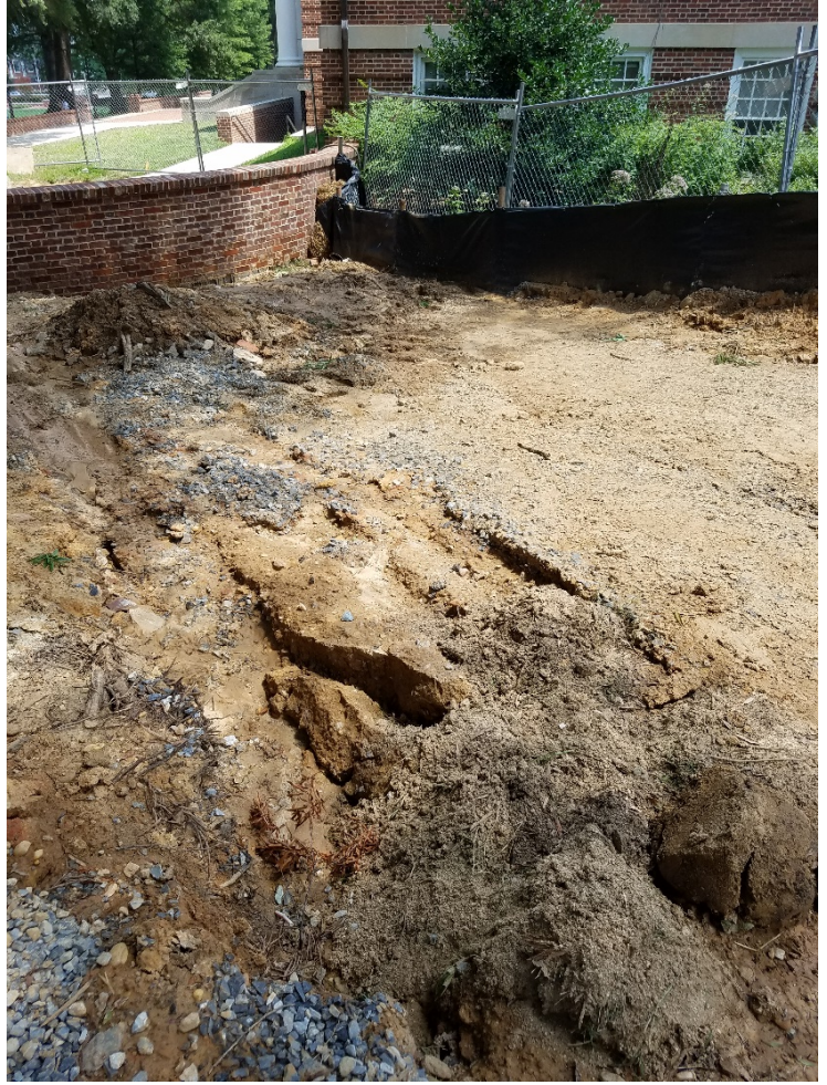
Between Francis Scott Key Hall (FSK) and Woods Hall, looking towards Woods Hall; large rill suggesting recent erosion. Storm drain is located on the right side of the pictured fence.
