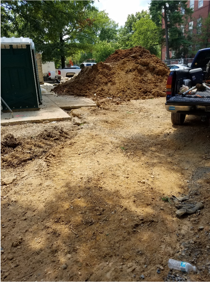
Between Francis Scott Key Hall (FSK) and Woods Hall, looking towards FSK; large soil pile uncovered and exposed to stormwater
