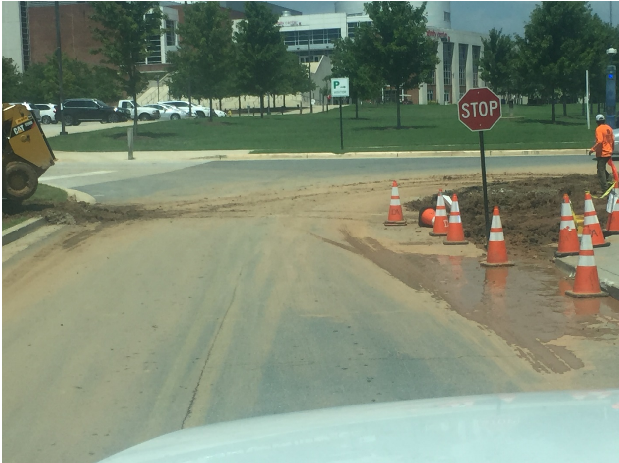
On Regents Drive looking north towards Xfinity Center, a small construction site without any BMPs discharging highly turbid, sediment laden water to Campus Creek
