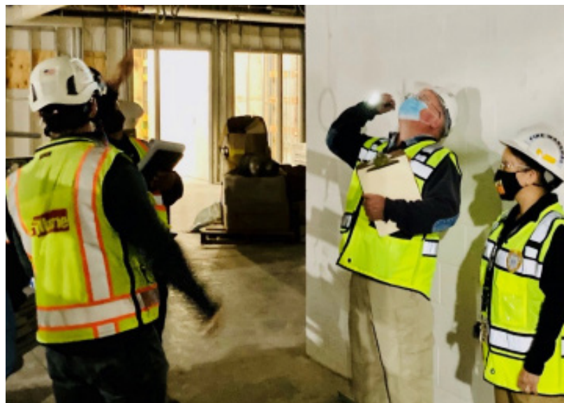
Fire Protection Engineers Keith Lippincott and Jessimay Llaneta conduct a site inspection at Cole Field House
