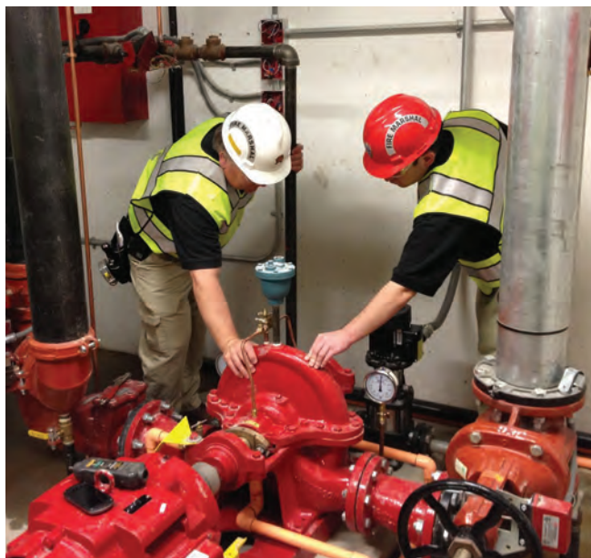
Inspecting a new fire pump
